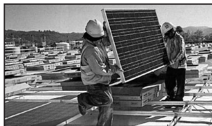
Photo 11 – Roofs acting as platforms should be designed not only to withstand the impact of constructoin crews unfamiliar with roofs, but also the equipment packaging, debris, and assembly areas.
