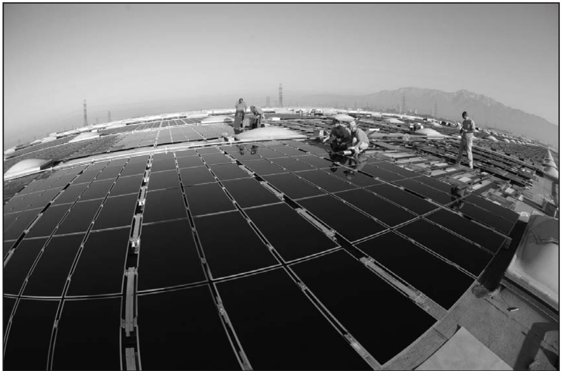
Photo 10 – This solar panel installation allows little room for maintenance of the roof surface below – a requirement of the roof warranty.
