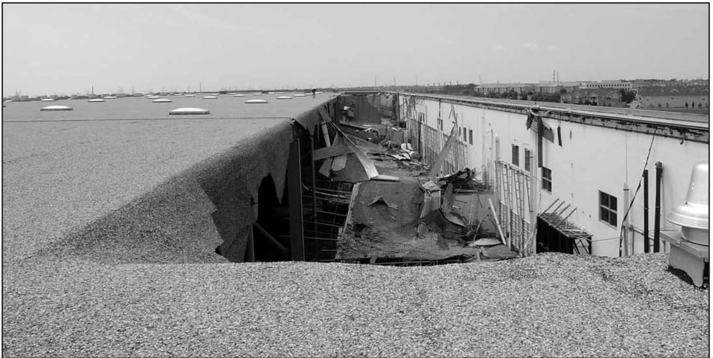
Figure 4 – An example of a typical roof collapse caused by inadequate roof drainage.
