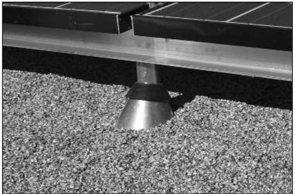
Figure 9 — Penetrating roof mount on gravel ballasted BUR. The same detail would be applicable to an embedded aggregate roof.
