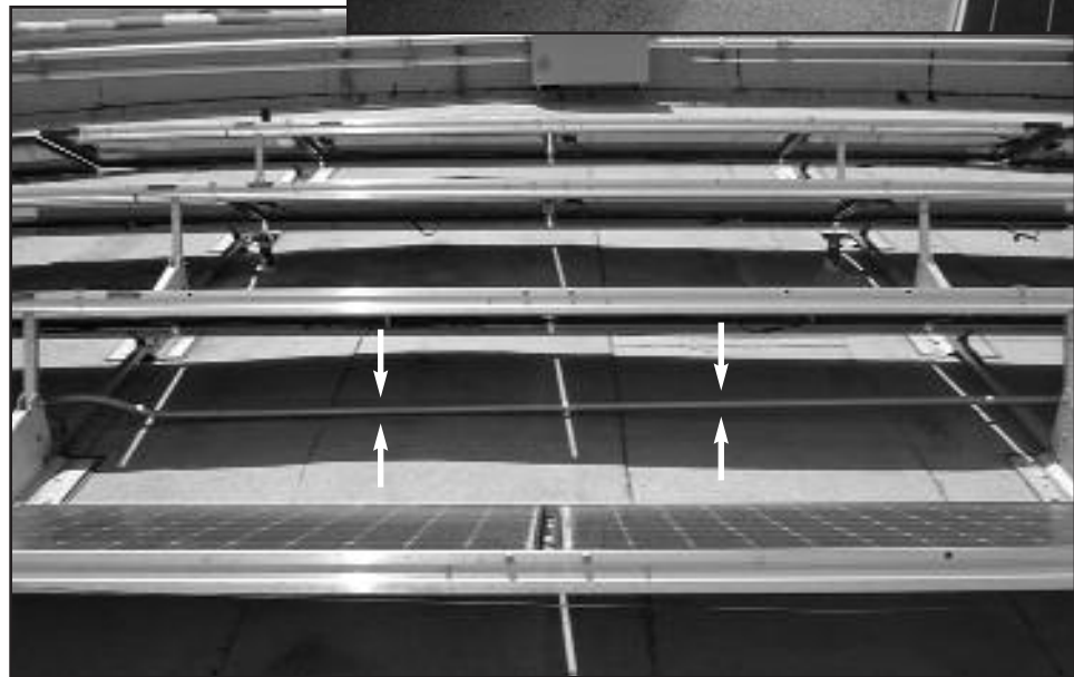
Figure 14 — Possible maintenance and safety issues caused by conduit lying on roof.
