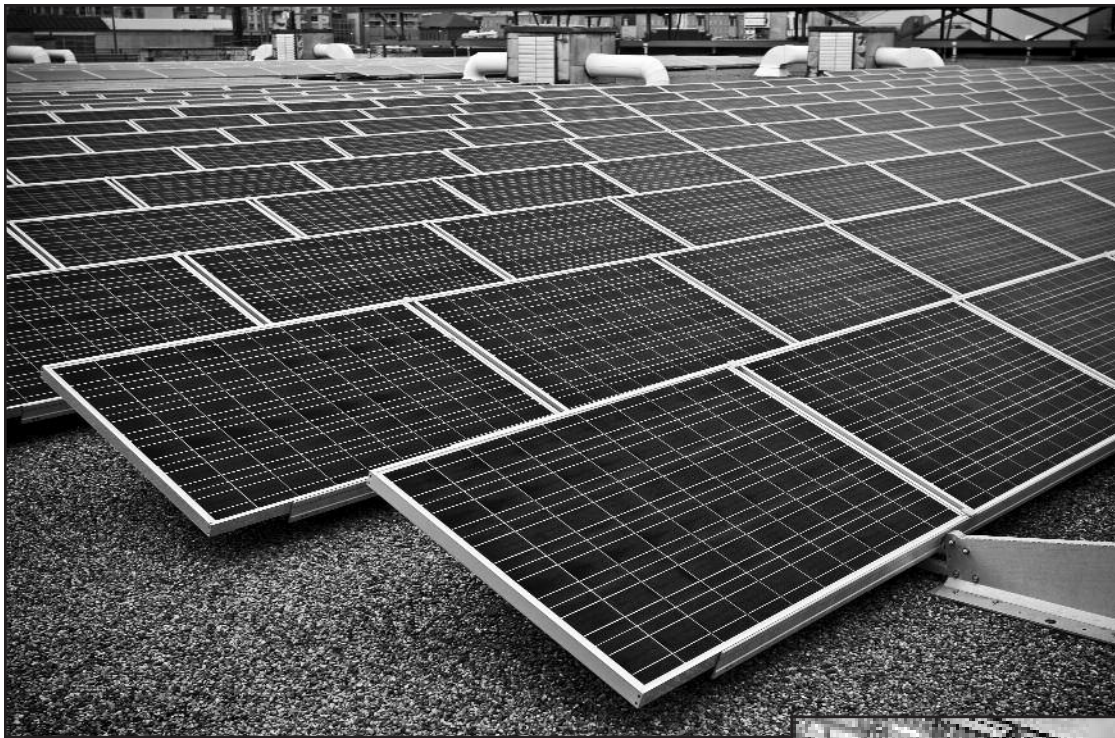
Figure 10 – Roof-mounted, ballasted solar panel system with polycrystalline panels. Note the limited clearance between the panels and the roof deck, possibly creating the need to remove the panels for the purposes of roof replacement or possibly even for normal roof maintenance, leak repair, or cleaning.
