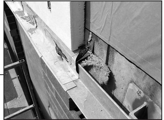
Figure 6 - Shelf angle on brackets.
