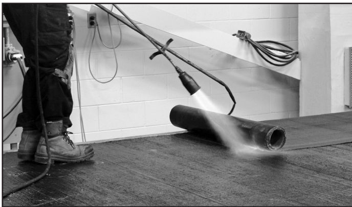
Figure 5C – A coat of primer, 100-400 gal/ft 2 (0.4-1.6 L/m 2 ), was applied on the top surface of the concrete deck. Base sheets were then torched to the concrete deck layer.
