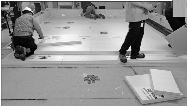
Figure 5E – An 18-in.- (457-mm-) high wooden parapet was installed all around the perimeter. Two layers of insulation were shipped and placed on top of the cap sheet.
