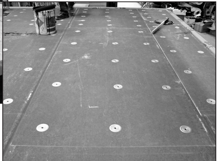
Figure 4B – Over the plywood, support boards were attached with 15 fasteners per board, using #14, 2\frac{3}{4} -in. (70-mm) fasteners and 3-in. (76-mm) metal plates.
