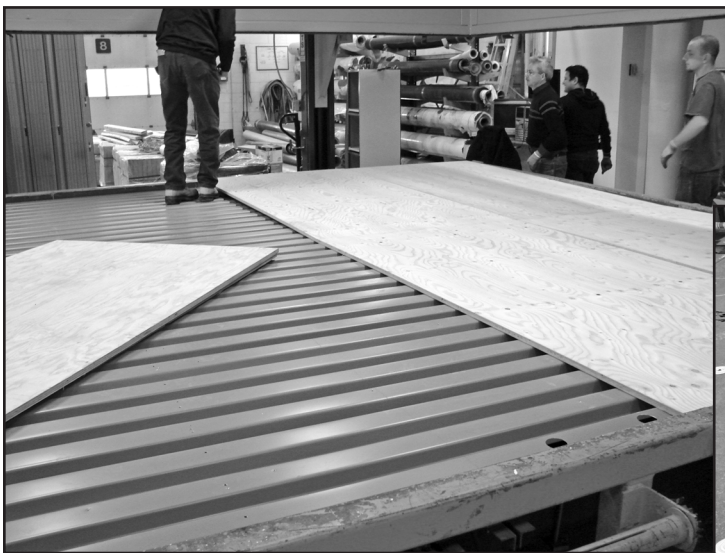
Figure 4A – \frac{3}{4} -in. x 4-ft. x 8-ft. (19 mm x 1219 mm x 2238 mm) sheets of plywood were placed on top the steel deck. Sheets were then attached with eight fasteners per board to steel deck using #14, 2\frac{3}{4} -in. (70-mm) fasteners.
