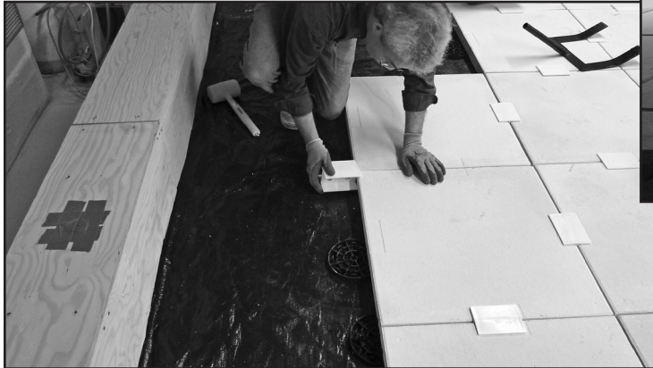
Figure 5G - Pavers were placed on the paver supports and interconnected with H clips.
