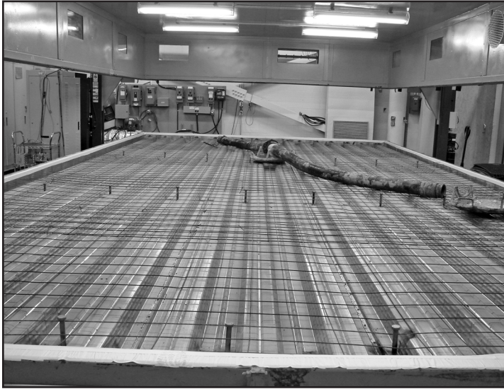
Figure 5A – Steel mesh was loose-laid on top of the welded steel deck.
