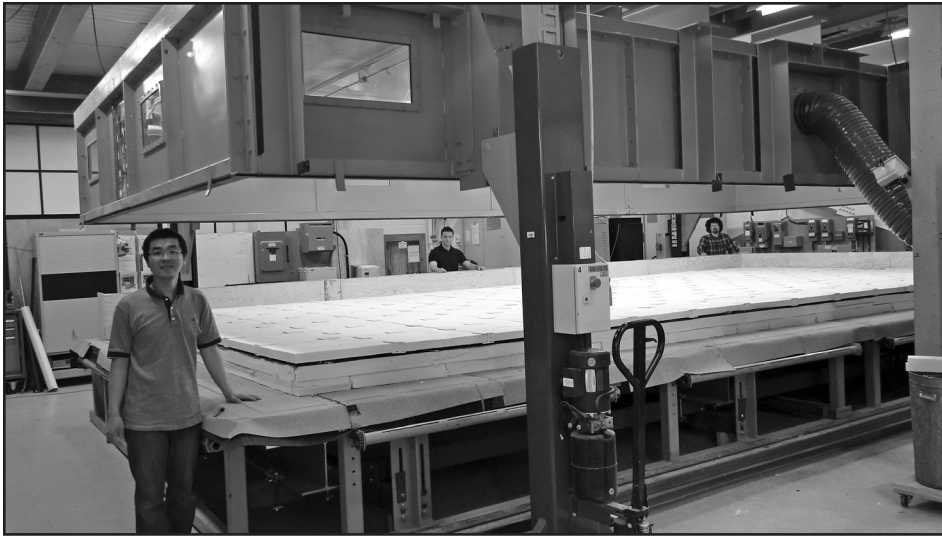
Figure 2 – A protected membrane system with a width of 16 ft. (4.9 m) and a length of 32 ft. (9.8 m) is ready for testing at the Dynamic Roofing Facility.
