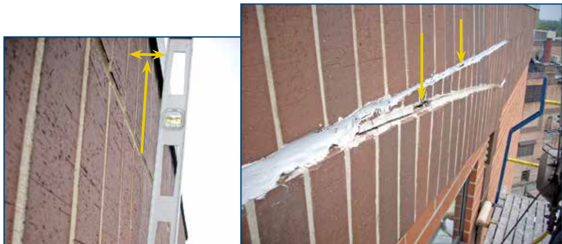
Figure 10 – Typical cracking of mortar joints at parapet wall in 2007.
