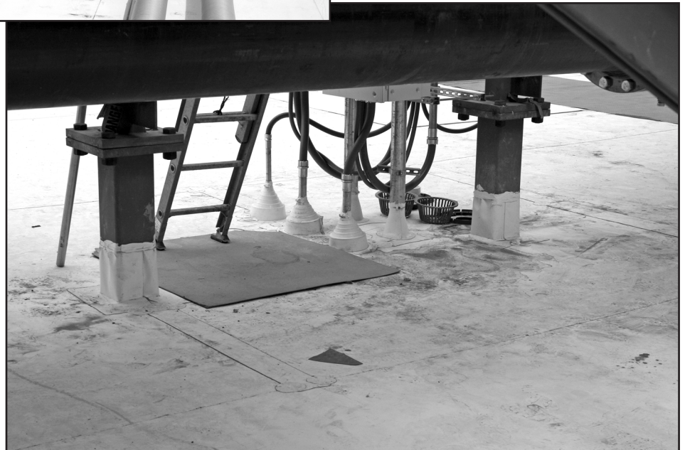
Figure 18 – Soiled roof condition (poor drainage).
