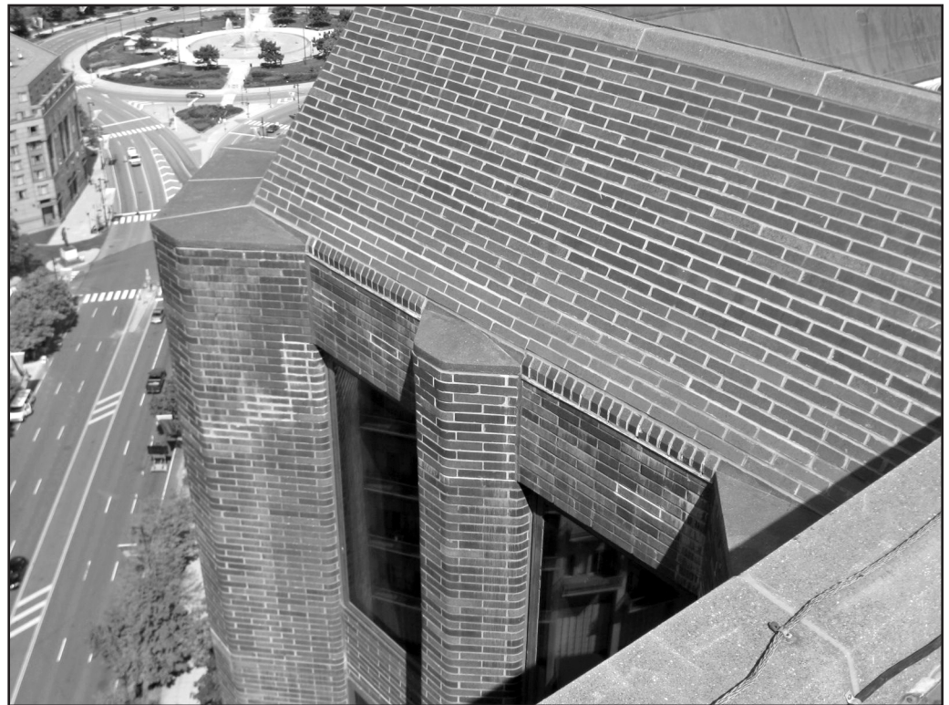
Photo 10 – Completed appearance at sloped wall, five-sided brick, and capstone. Contrast with soiled, unrepaired appearance below.
