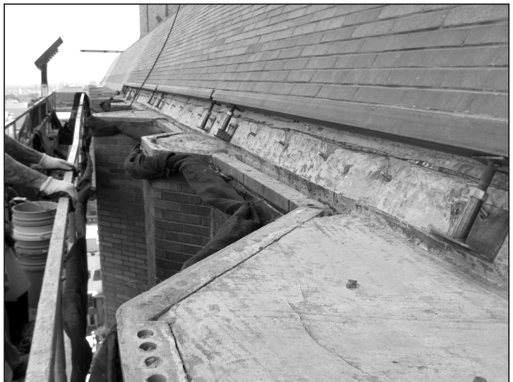
Photo 8 – Sloped brick supported with temporary steel and fabricated clips at angle fasteners.
