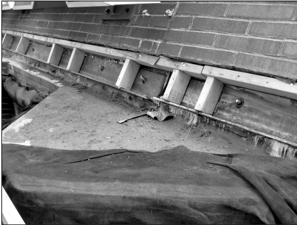
Photo 7 – Conditions at the base of the sloped wall created difficulties in addressing lintels and installing new through-wall flashing.
