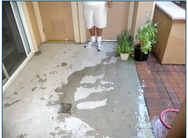
Figure 22 – Water flows from the door even though it never flows to it.
