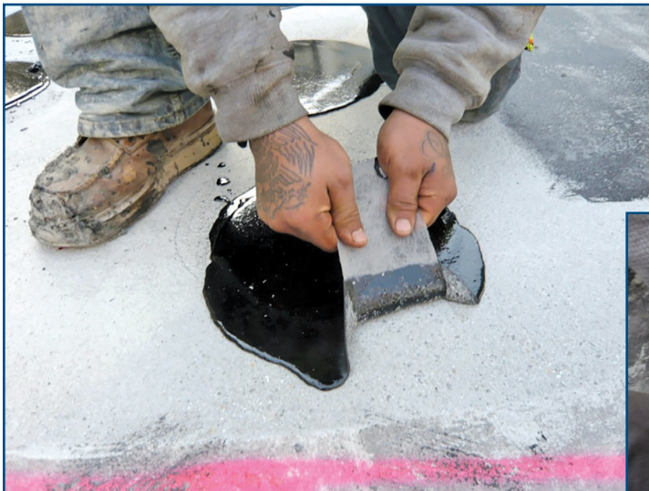
Figure 26 – This sample exhibits failure in adhesion due to a water-based primer that was used in the application that was not curing due to cold temperature.
