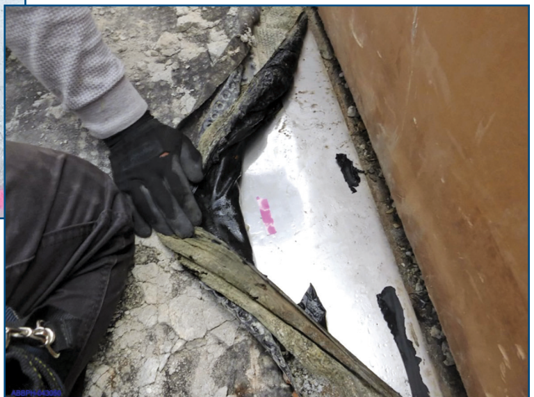
Figure 27 – Adhesion failure of cold-fluid-applied membrane to stainless steel flashing due to lack of proper priming and prep work.
