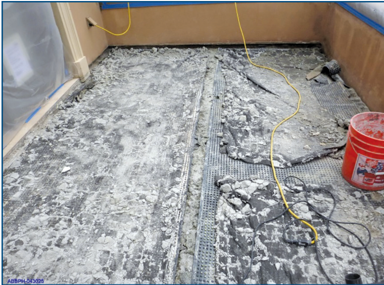
Figure 24 – On this wood-framed balcony deck, the drain mat was discontinuous down the center of the deck. This resulted in water not properly flowing and ponding on the upslope side of the discontinuity.
