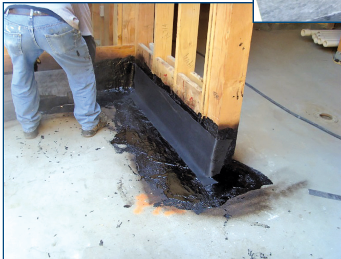
Figure 13 – HRA challenge – flashing buildup.
