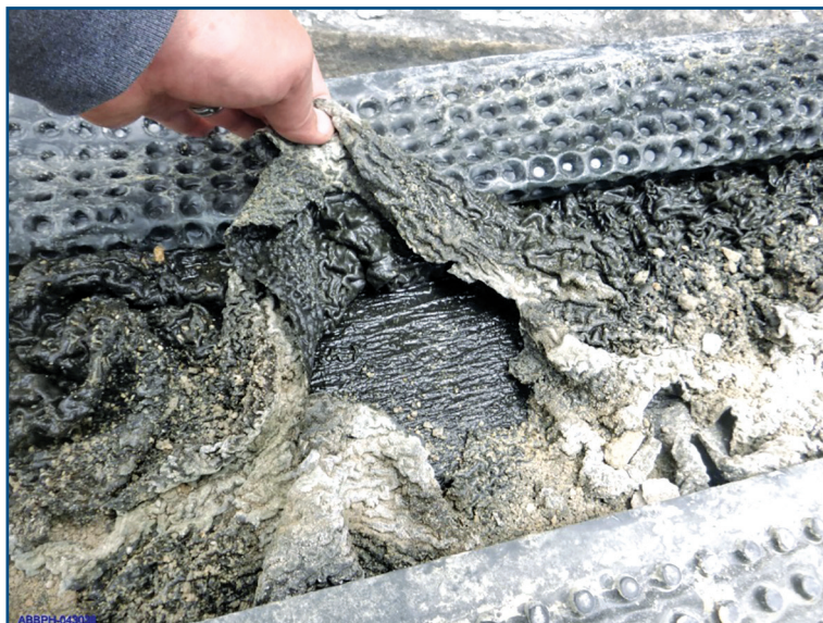
Figure 16 – Modified polyurethane membrane is swollen and looks like the texture of a brain and is referred to as “brainiac.” Prolonged immersion of the membrane results in swelling and water absorption far beyond the manufacturer’s published results.
