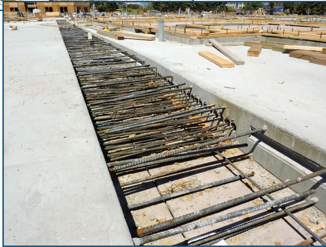
Figure 4 – Post-tensioned reinforced concrete slab under construction. Also common in steel structures is steel pan deck, with mild steel-reinforced concrete. Prior to the adoption of reinforced concrete, the two-way flat plate and one-way slab-over-beam systems were common; however, they are not used much anymore.
