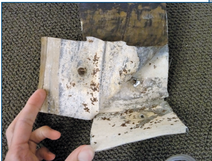
Figure 18 – Corrosion of galvanized sheet metal flashings under 90 mils of fluid-applied membrane.
