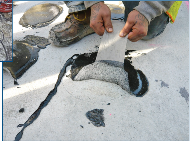
Figure 25 – Interestingly, the failure mode is in cohesion of the concrete, as opposed to adhesion of the membrane. The concrete slab surface had improperly cured and was soft and chalky.
