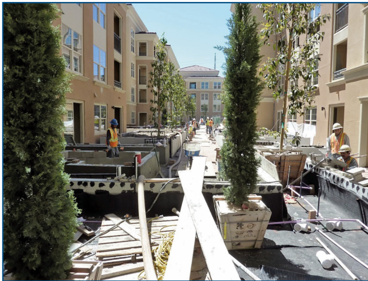
Figure 2 – Typical podium under construction with waterproofing complete inside of planters. Due to the heavy construction traffic, waterproofing membrane is phased and installed last, before the wearing course.
