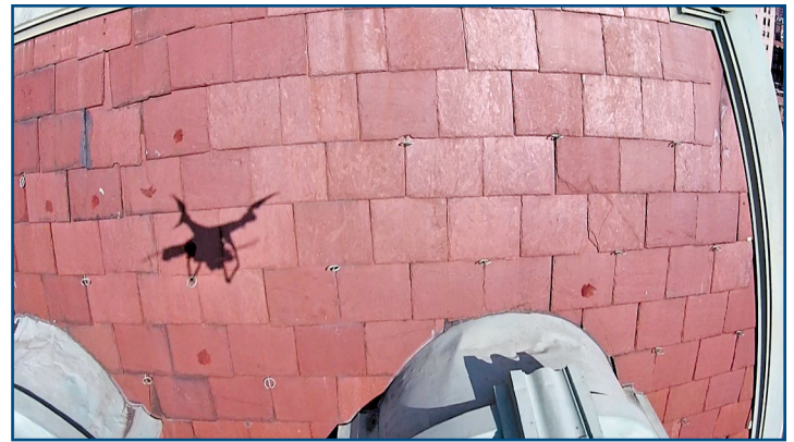
Figure 12 – Image from drone of steep-sloped, mansard roof area of educational building in Figure 5.
