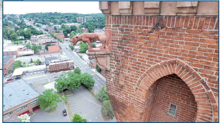
Figure 17 – Image from a drone. Crack in brick masonry is visible.
