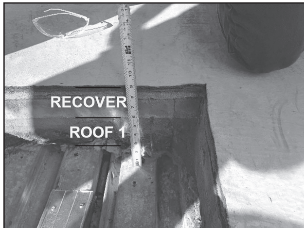
Figure 2 – Roof re-cover scenario where an existing roof is removed and the metal deck receives a new mechanically fastened roofing system.
