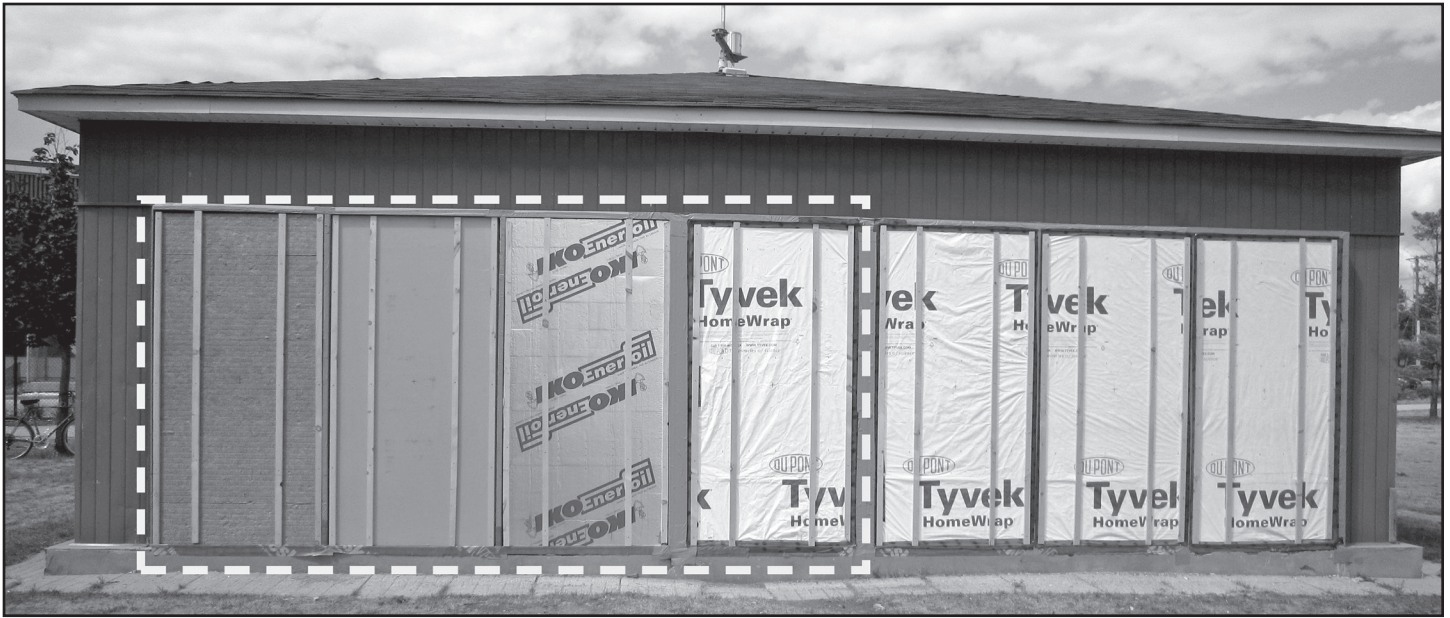
Figure 6 – Exterior-insulated (three on left) and datum (one at middle) test wall assemblies before siding.
