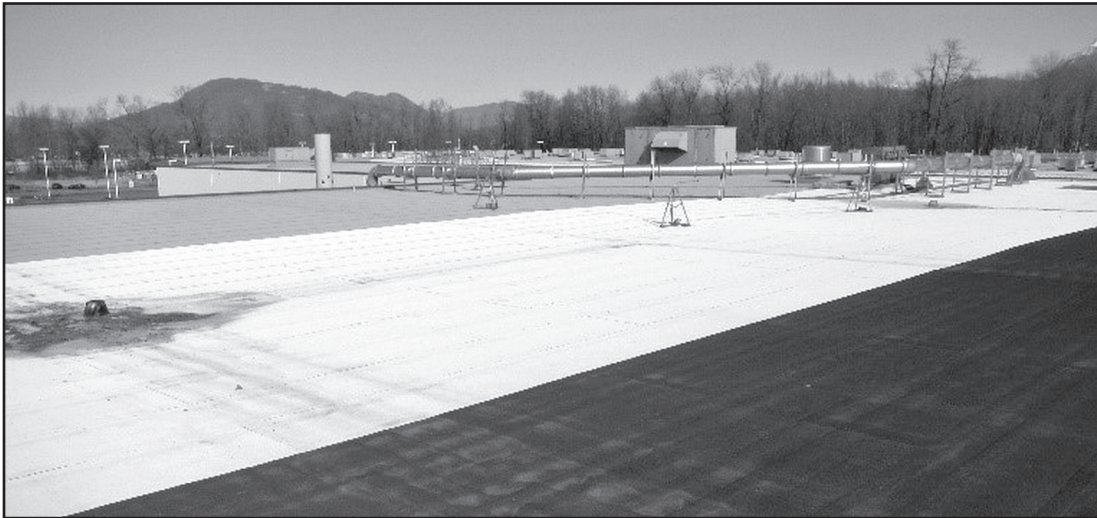
Figure 2 - Photo of test roof area showing three different roof membrane colors: black, white, and gray.
