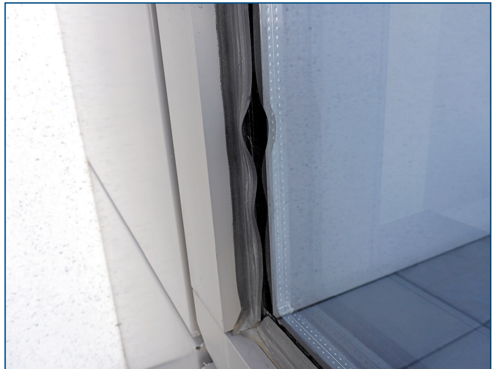
Figure 3 – Example of gasketing failure.
