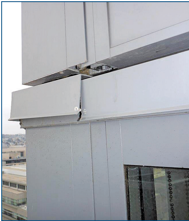
Figure 11 – Sample of trim cover failure.
