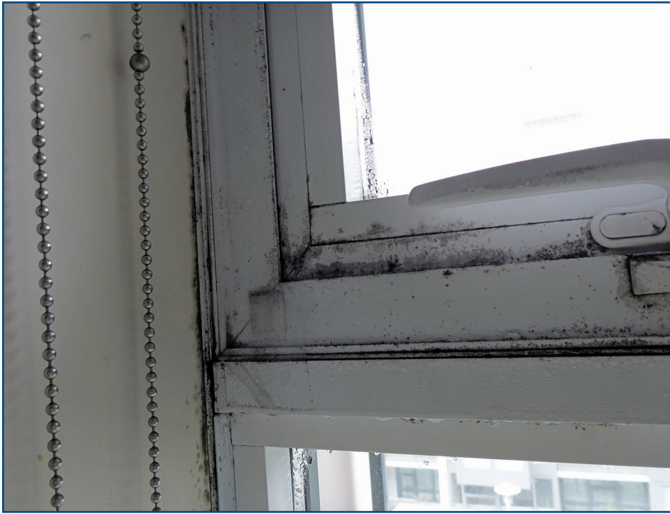
Figure 8 – Example of condensation failure.
