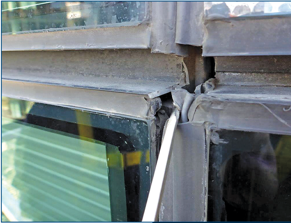
Figure 4 – Path of water intrusion over IGU glass edge.
