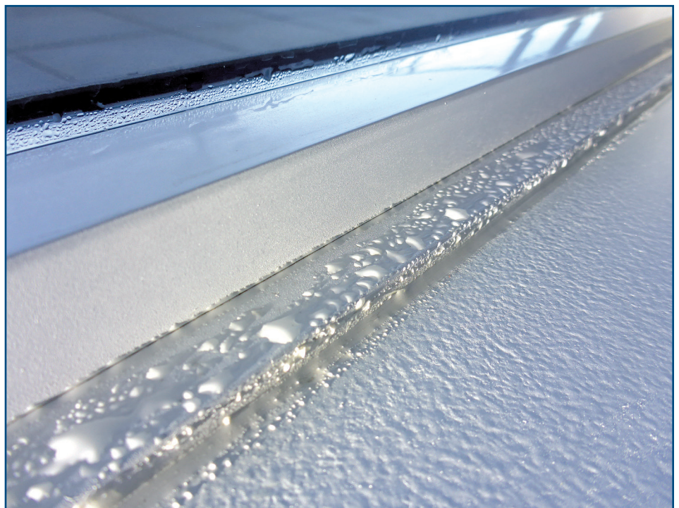
Figure 10 – Condensation on an interior window surface.
