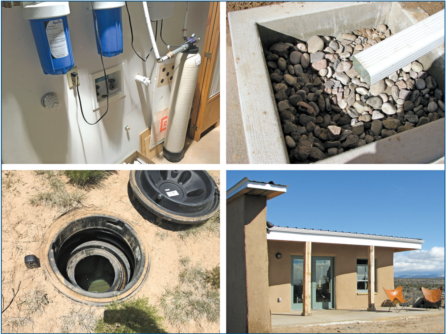
Figure 15 – Top left: Micron and UV filters; top right: catch basin and rock filter; bottom left: buried cistern on south side of house; bottom right: gutters on western façade.
