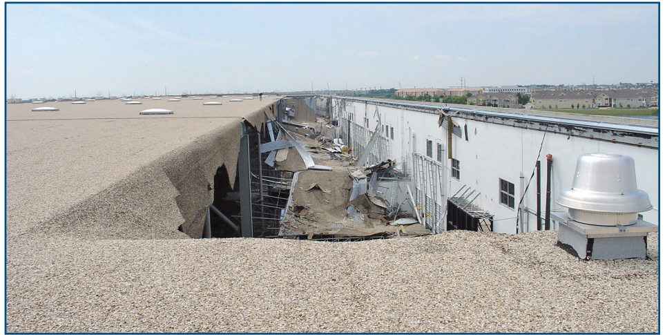
Figure 1 – A typical drainage-related collapse of a low-slope roof. Photo by Stephen Patterson.
