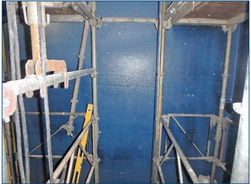
Figure 15 – Note the limited physical access between the scaffolding and shaft wall plane. Note the continuous blue air and vapor barrier.
