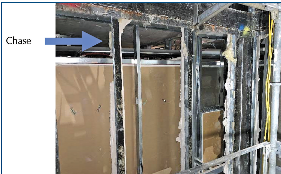
Figure 14 – Fire-rated shaft wall has been removed, but framing remains. Note the ceiling chase area that extends across the ceiling of the ninth-floor units creating challenges to maintain negative pressurization.
