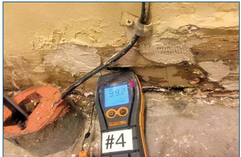
Figure 3 – Telephone closet at floor line. Note moisture reading during summer proposal visit.
