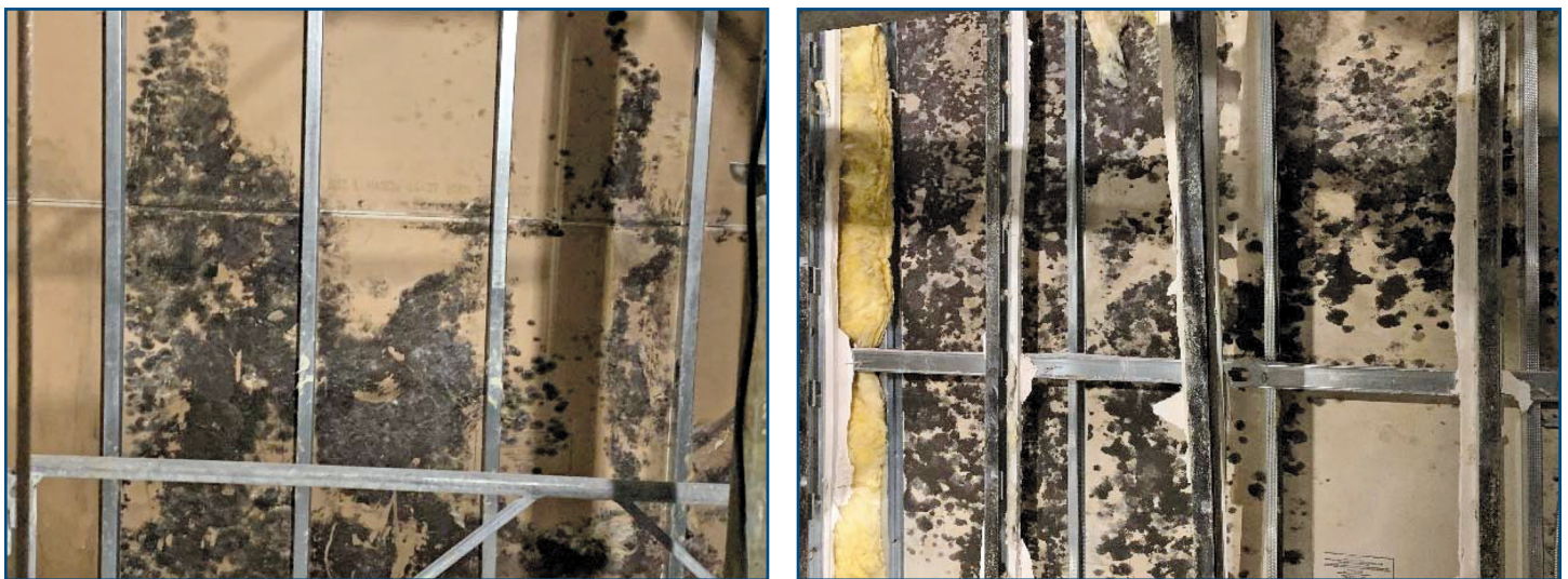
Figures 10A and 10B – Organic growth was encountered at various locations on the cavity side of the demising partitions that required abatement.
