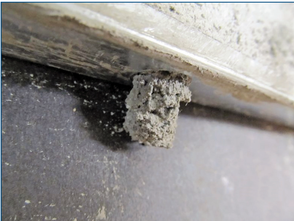
Figure 10 – Mortar extrusion through weep screed drainage surface perforation (weep holes).
