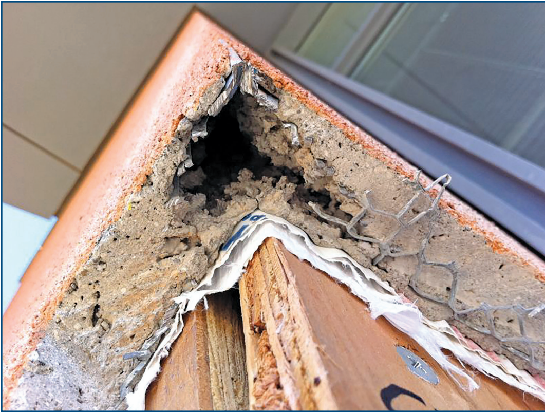
Figure 2 – Corner bead lathing accessory—hollow because it was incorrectly plastered.
