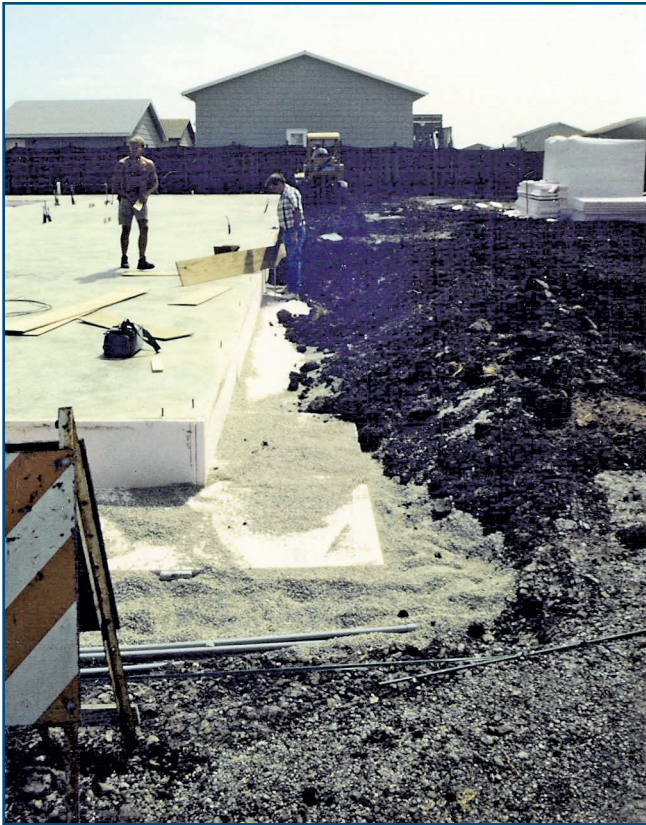
Figure 7 – Example of a frost-protected shallow foundation using foam sheathing CI (16-in.-deep thickened-edge slab built in Fargo, ND).
