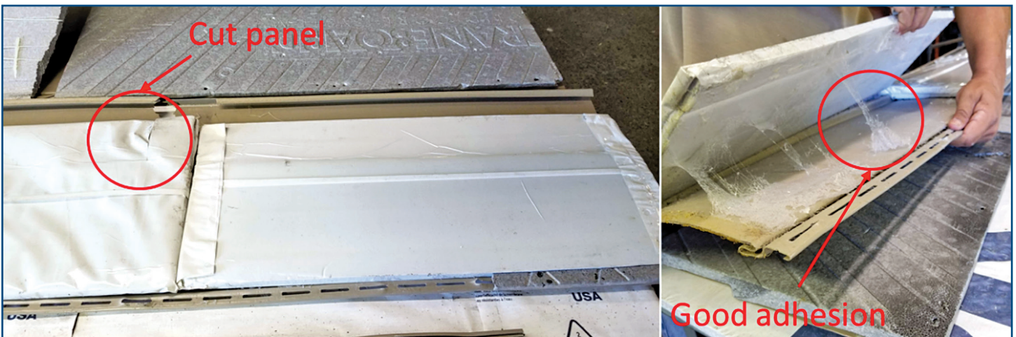
Figure 8 – Siding autopsy. Panels still fully adhered to siding.
