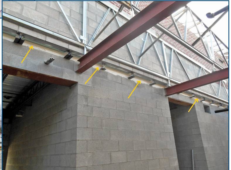
Figure 19 – Fire Station A. View of steel-supported second-story masonry veneer cladding and large potential air leaks, which were discovered and sealed during construction at the base of the open cavity above the first-floor ceiling space.
