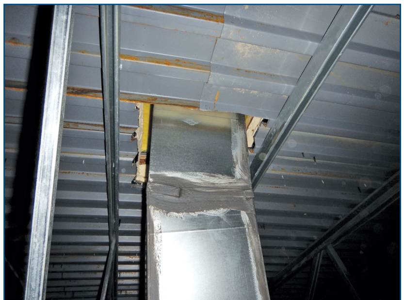
Figure 13 – Fire Station B. View of typical roof deck penetration for a duct where the roof deck penetration must be sealed on the top side of the deck to prevent air infiltration/exfiltration via the compact ventilated roof assembly.
