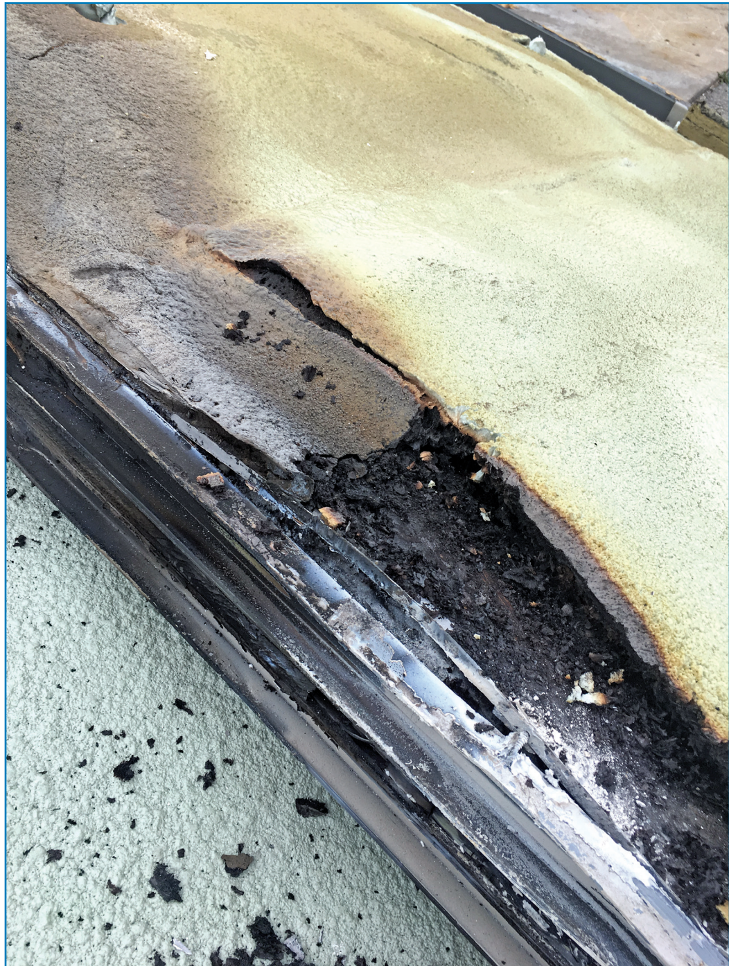
Figure 6 – View of localized charring of spray foam at vertical above-window opening.
