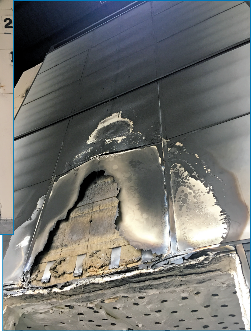
Figure 5 – Exposed mineral-wool insulation above window opening.
