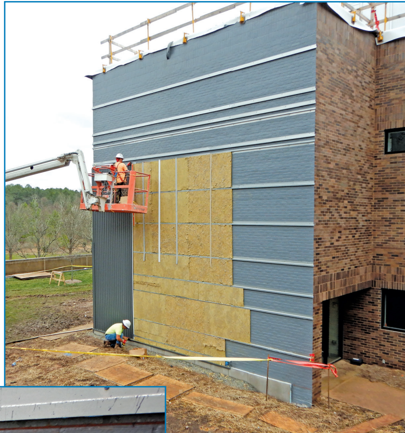
Figure 10 - Ongoing work where the liquid-installed air barrier is visible, as well as horizontal Z tracks and thermal insulation prior to installation of metal wall panels.
