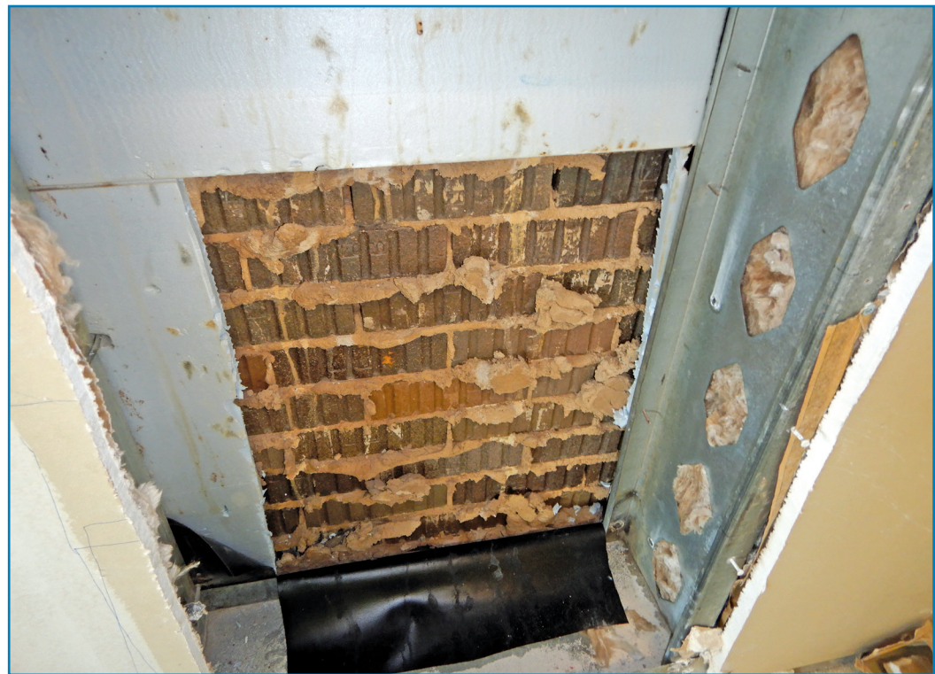
Figure 5 – Forensic study image where the brick cladding was inspected from the inside of the building by removing interior finishes and sheathing. Note through-wall flashing at bottom of photo.
