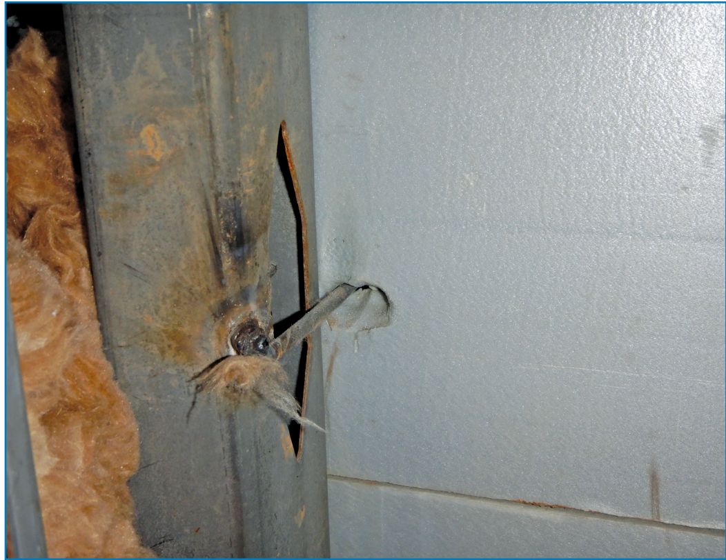
Figure 6 – Forensic image of one of the methods used, fastening brick cladding anchors to the steel studs where the anchors were field-welded in place; note large hole melted in the foam sheathing.
