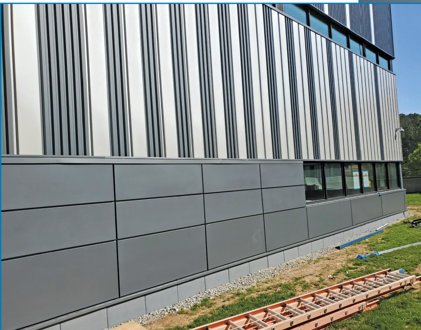
Figure 13 – Completed wall depicting various metal panel types as well as insulated concrete-coated rigid insulation panels at base of wall.
