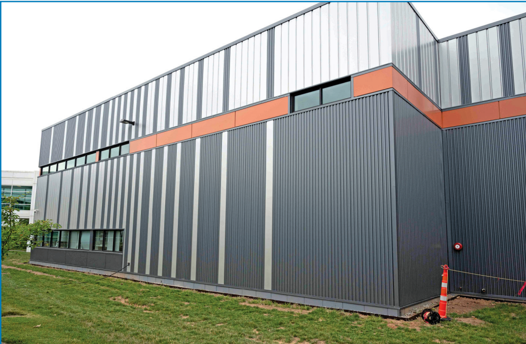
Figure 14 – Completed end wall with custom colors and variation of metal building wall panels.
