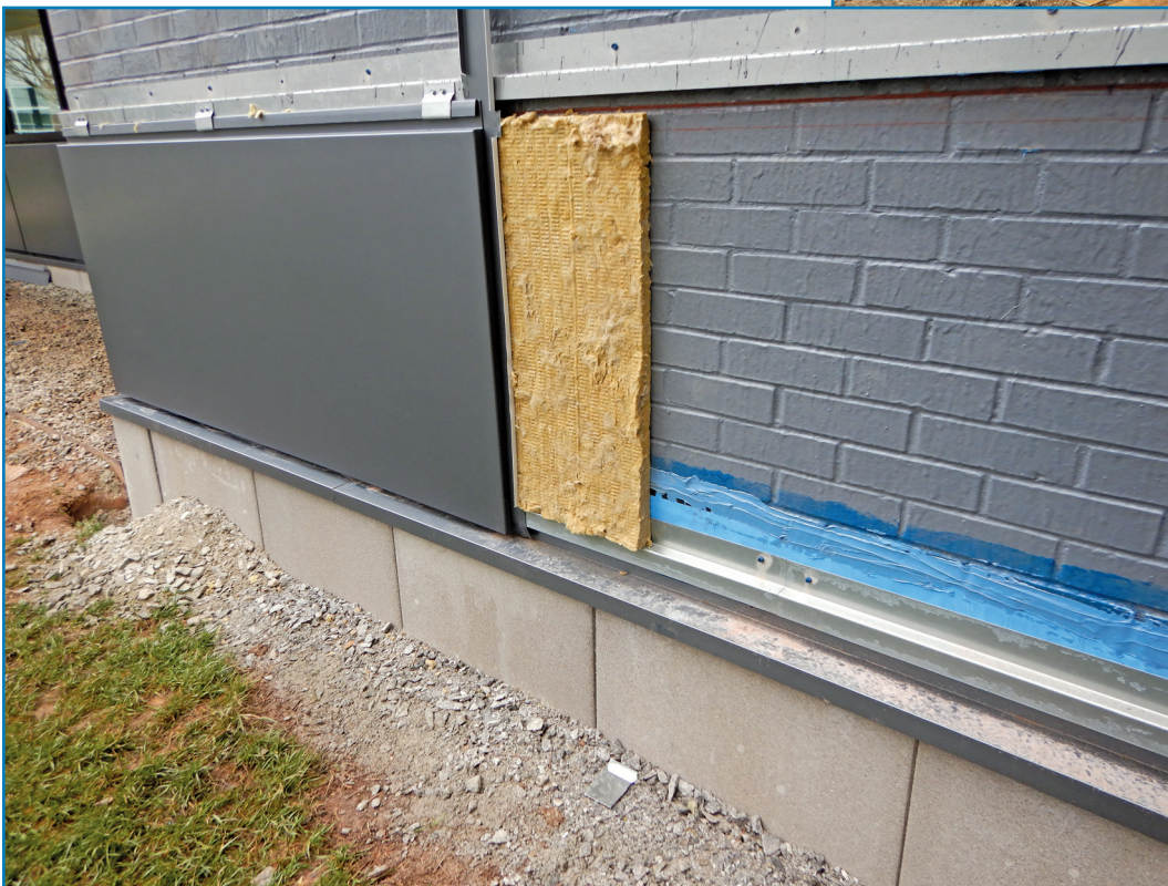
Figure 9 - Base-of-wall condition where through-wall flashing is secured to the primed air-barrier membrane to flash out water before the base-of-wall insulated concrete panels below.
