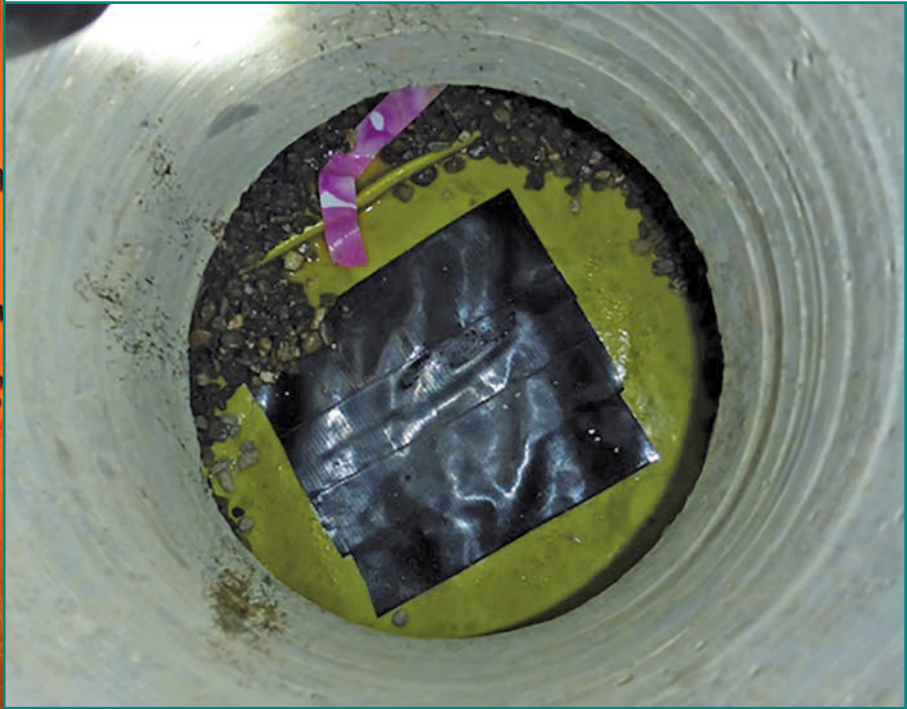
Figure 2 – Water under concrete slab.
