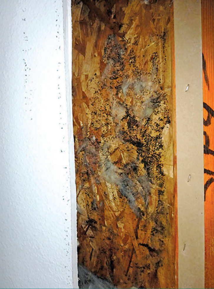
Figure 1 – Decay on back side of OSB sheathing.
