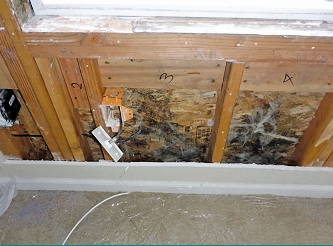
Figure 8 – Biological growth on back side of wood sheathing after removing gypsum board.
