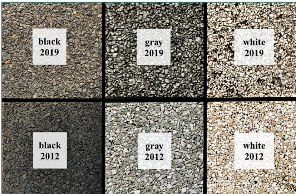
Figure 7 – Roof membrane samples comparing original 2012 (bottom) vs. aged 2019 (top) for black, gray, and white membrane colors.
