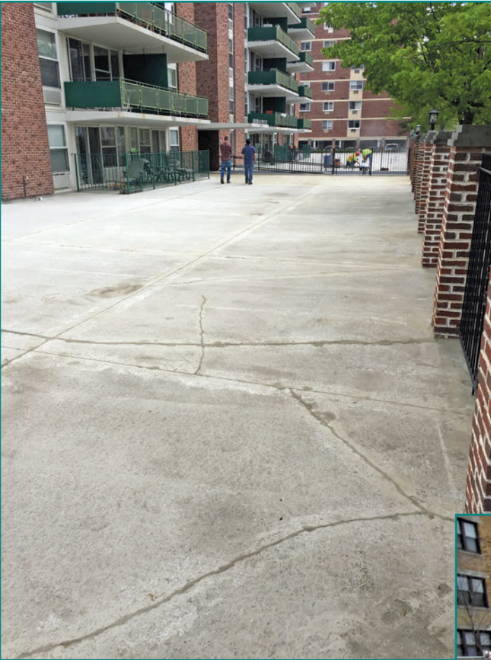
Figure 4 – Case Study 1 plaza with cracked and unsightly concrete paving surface.
