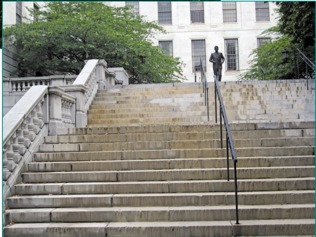
Figure 8 – Staining and efflorescence at stairs.
