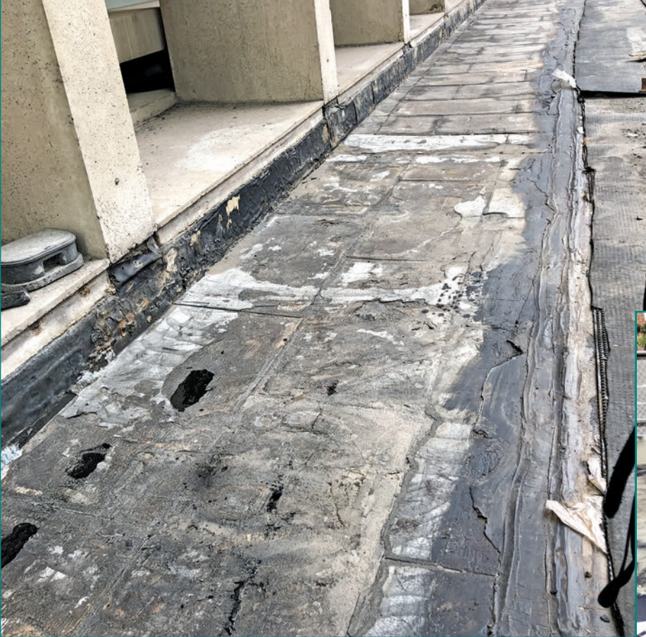
Figure 1 - Aged self-adhered sheet membrane exposed in plaza waterproofing system.
