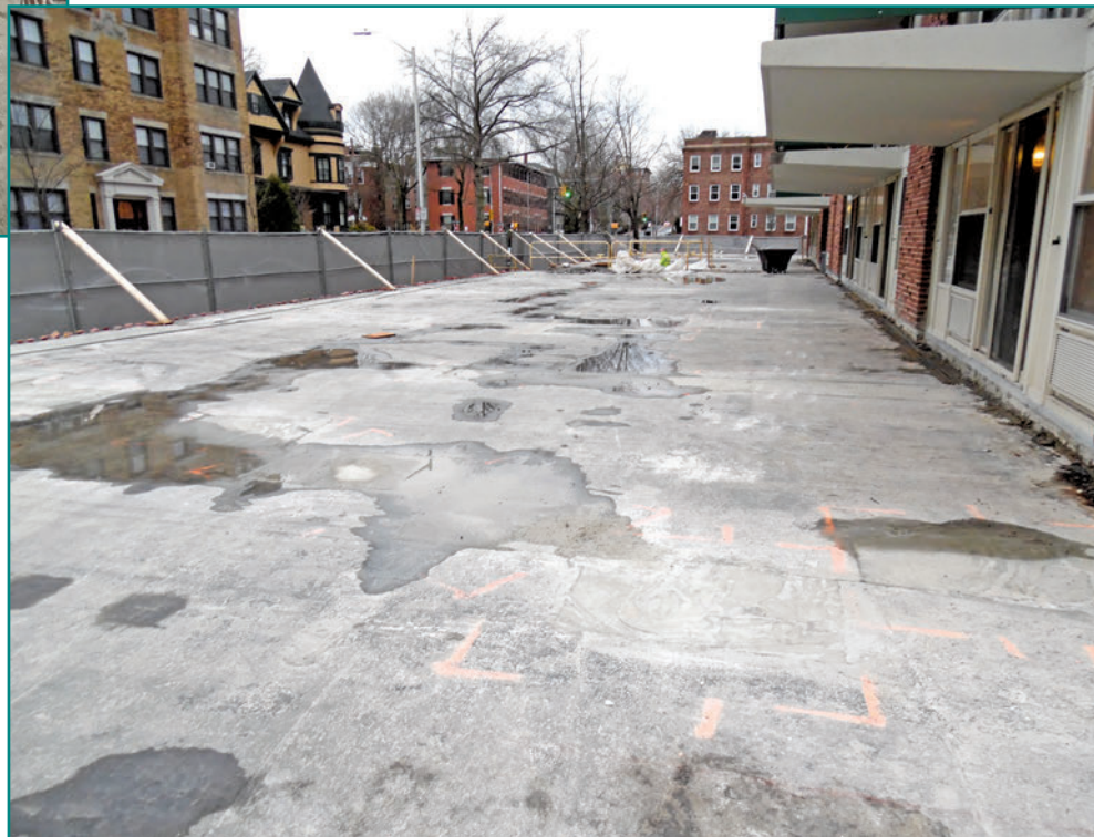
Figure 5 – Concrete structural slab lacks slope to drain and water ponds on the surface.
