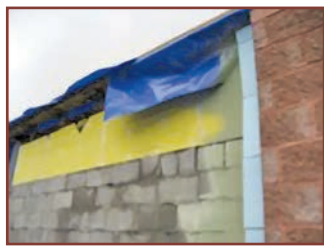
Figure 1. Roof-to-wall transition “done incorrectly” with noncompatible materials and numerous voids.
