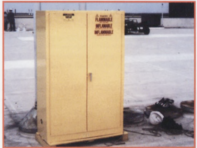
Flammable materials should be properly stored. Fire cabinet is secured to roof penetrations and is easily identifiable as containing flammable materials.
