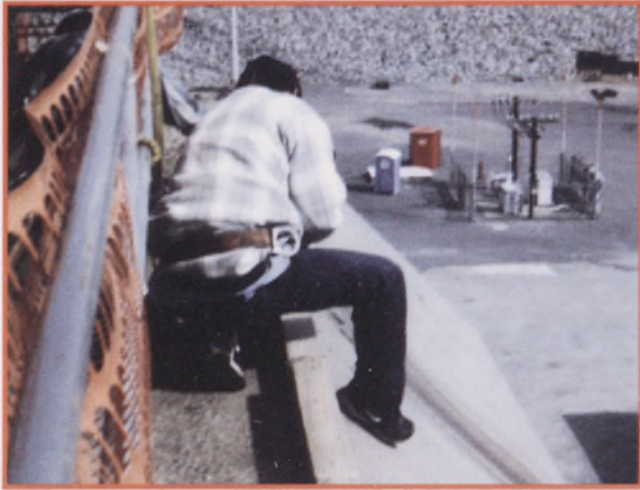
This worker is improperly using a safety belt for fall protection. Fall prevention and fall protection are different and require different equipment and procedures. If you are going to be exposed to a fall hazard, you must know the difference in order to protect yourself.
