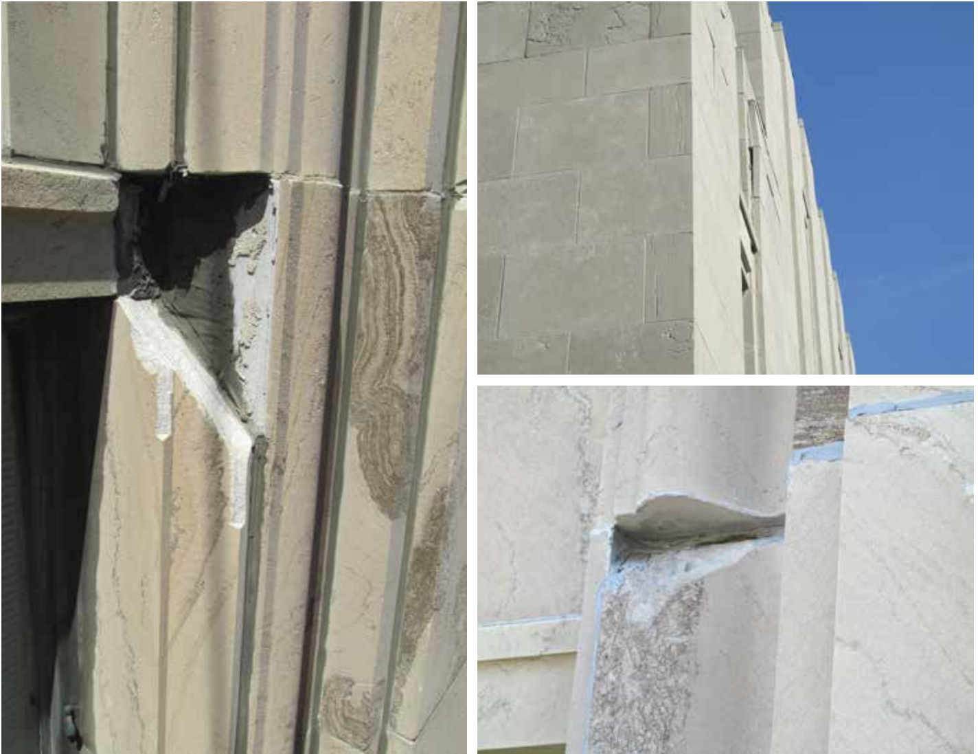
Figure 4. Examples of cladding distress observed.
