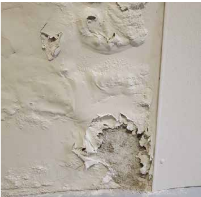
Figure 2. View of moisture-related damage to interior finishes.
