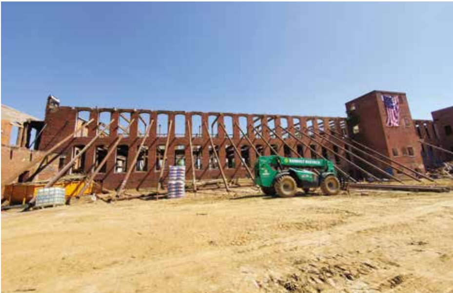
Figure 1. Overview of previous industrial mass masonry structure during construction of adaptive reuse project.
