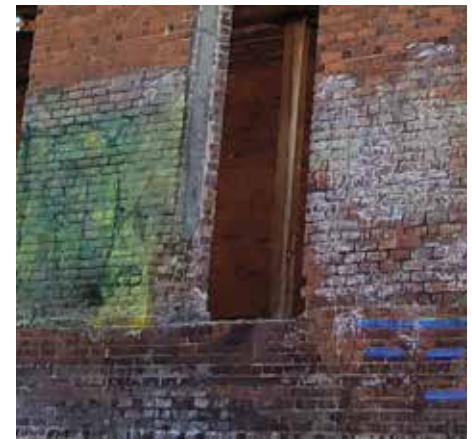
Figure 5. Representative view of masonry requiring restoration.
