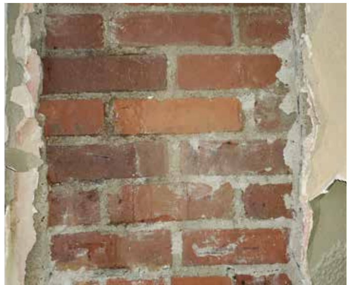
Figure 7. Representative view of damp portion of wall with water weeping from anomalies at the interior masonry surface.
