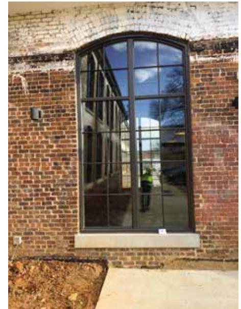
Figure 10. Representative view of new fenestration installed in existing mass masonry wall opening.
