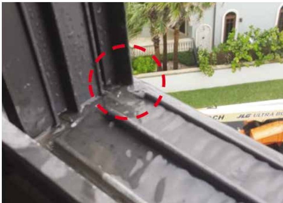
Figure 1. Base of sliding window was previously blocked and allowed water accumulation.
