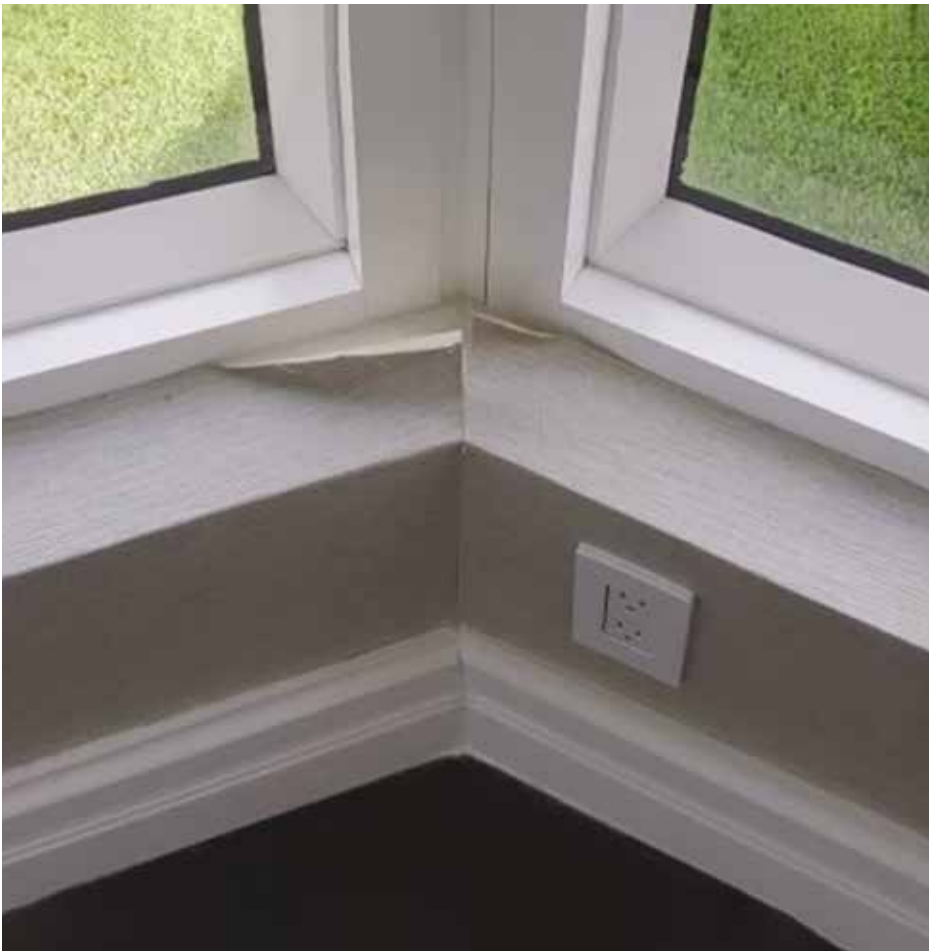
Figure 6. Distortion at window.
