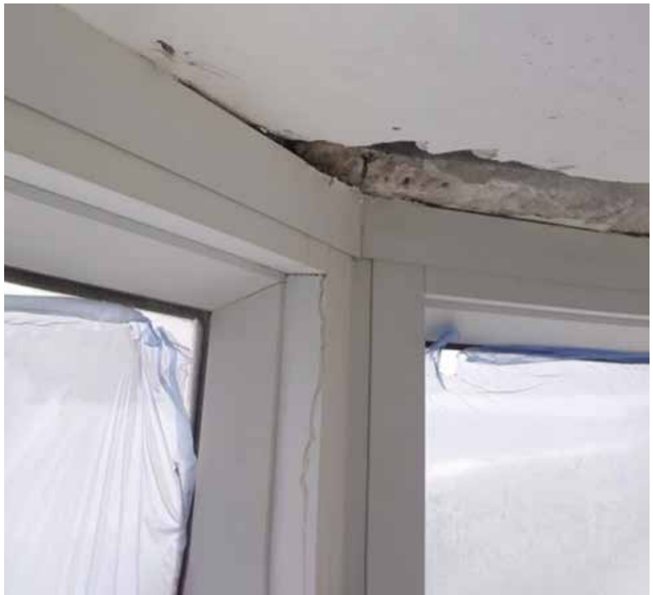
Figure 4. Red stains reveal compromised conduit not window assembly.
