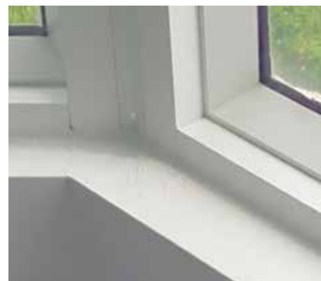
Figure 3. Improper assembly at the joining of window systems.
