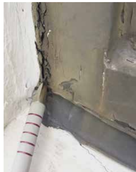
Figure 2. Aged sealant conditions around a window.
