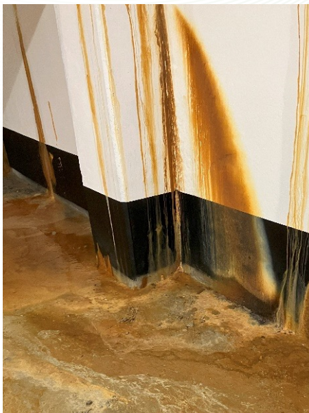
FIGURE 5. Water infiltration through foundation wall at column location.
