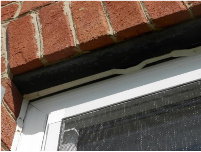
PHOTOGRAPH 2. Sealant separation at a window secured to wood framing due to shrinkage of the wood framing and expansion of the brick veneer. Photo from Rimkus Archives.
