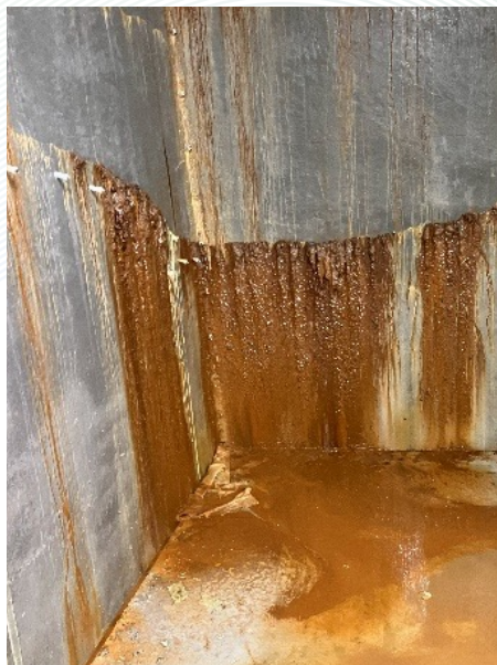
FIGURE 6. Water infiltration through foundation wall cracks at corner.
