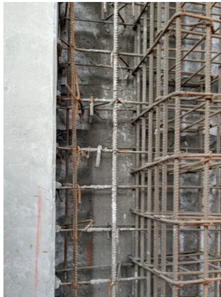
FIGURE 3. Shotcrete overspray on sheet membrane after form work was removed. No additional overspray removals were expected.
