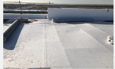
FIGURE 1. Failed roof assembly after heavy wind conditions
