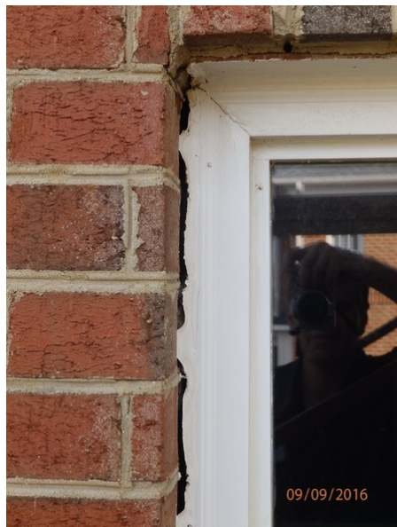
PHOTOGRAPH 14. Joint separation at the window in a bowed brick veneer wall. Photo from Rimkus Archives.
