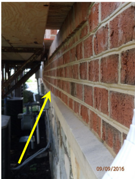
PHOTOGRAPH 13. Bowed brick veneer. Photo from Rimkus Archives.
