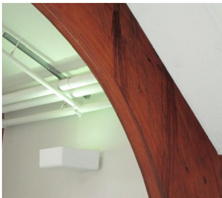
FIGURE 3. Staining from the roof on the interior structure.
