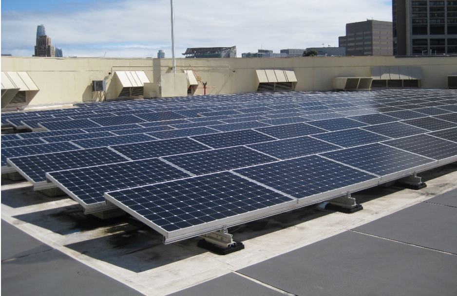
FIGURE 1. Example rooftop PV arrays on racks.
