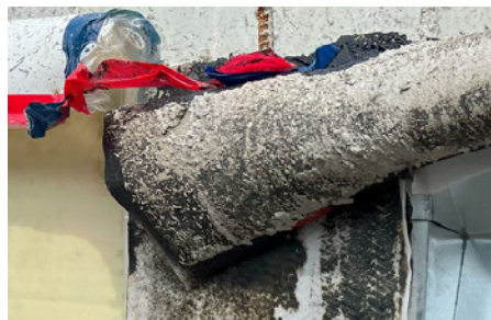
FIGURE 18. Concrete Splatter is found on overlap joint above the concrete pour.
