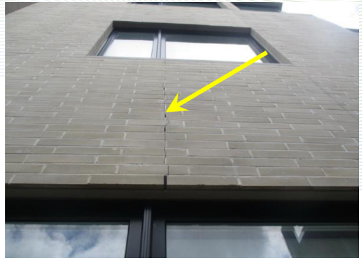
PHOTOGRAPH 8. A vertical crack. Photo from Rimkus Archives.
