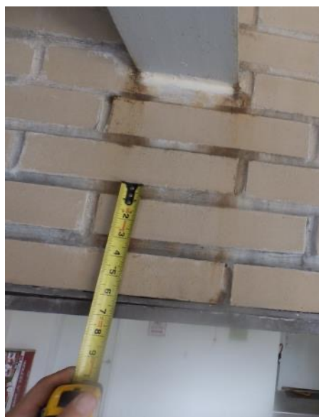
PHOTOGRAPH 16. Efflorescence on the brick-and-mortar joint surfaces. Photo from Rimkus Archives.
