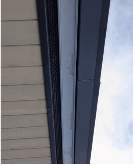
FIGURE 13. Photograph of water within the light fixtures at the edge of the soffit.
