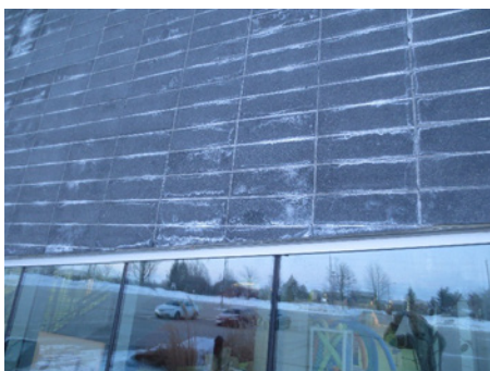
FIGURE 16. Around the windows, there was greater mortar damage and efflorescence as a result of the lack of deficient air barrier details.
