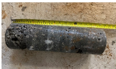
FIGURE 8. Extracted core from foundation wall showing unconsolidated concrete.
