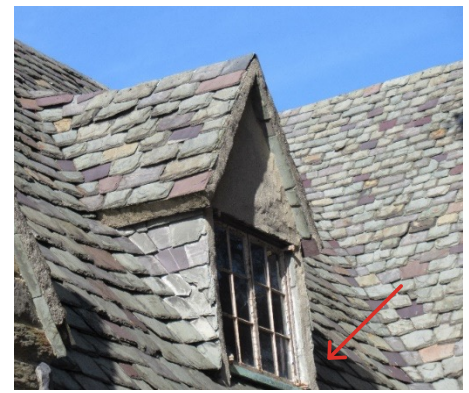
FIGURE 2. Install sensors in the north slope under shade (wintertime), red arrow indicates the sensor location.
