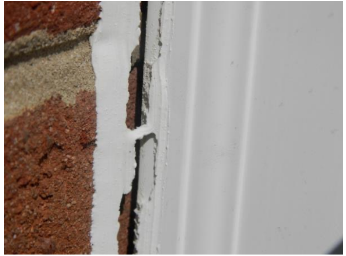
PHOTOGRAPH 3. Sealant separation at a window secured to wood framing due to shrinkage of the wood framing and expansion of the brick veneer. Photo from Rimkus Archives.
