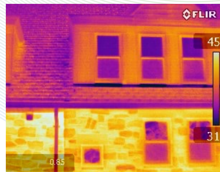
FIGURE 5. Exterior infrared image of a dormitory building at a college in Philadelphia, Pennsylvania, originally built 1981.
