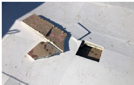
FIGURE 3. Exploratory opening investigation conducted post failure
