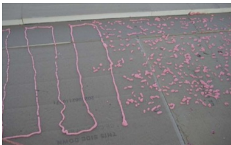
FIGURE 2. Poor installation practices observed and corrected
