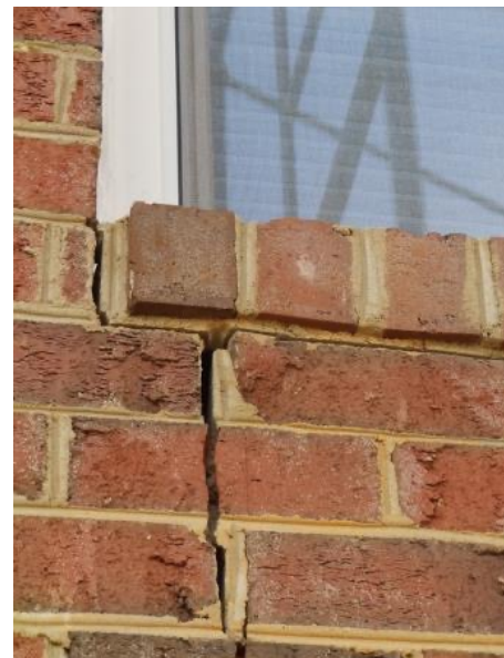
PHOTOGRAPH 15. A vertical crack in a bowed brick veneer wall. Photo from Rimkus Archives.
