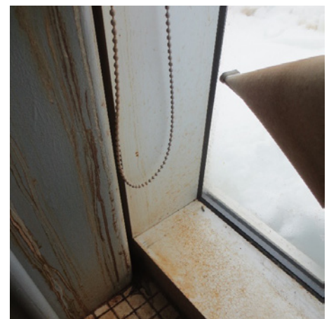
FIGURE 8. Staining inside the pool area running down steel columns from the parapet.
