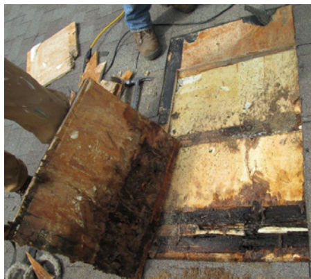
FIGURE 4. Rotting of the wood at the exterior of the roof assembly.
