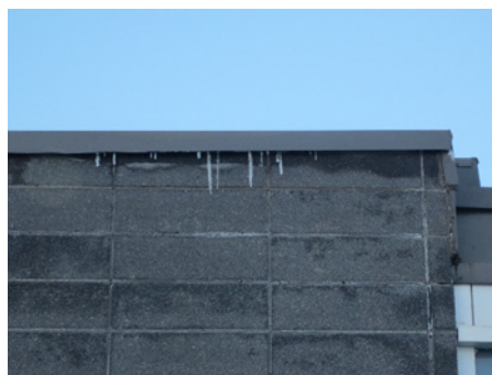
FIGURE 17. At the top of the wall, icicles, wetting, efflorescence, and mortar damage were all present as a result of air leakage.
