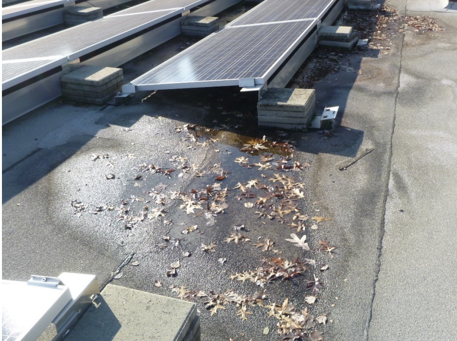
FIGURE 7. Localized deflection and ponding under ballasted PV assembly.
