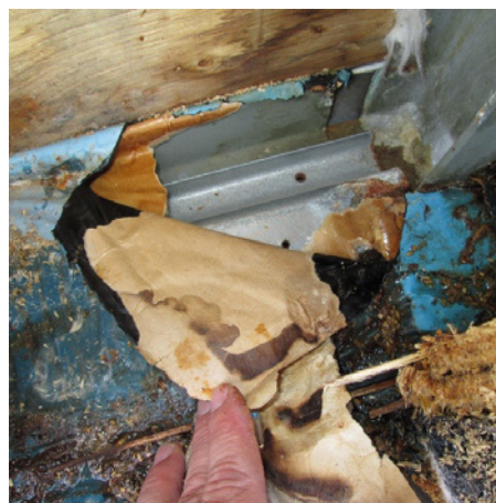
FIGURE 7. Water accumulation and damage in the parapet, and the backer observed on the Blueskin air barrier.
