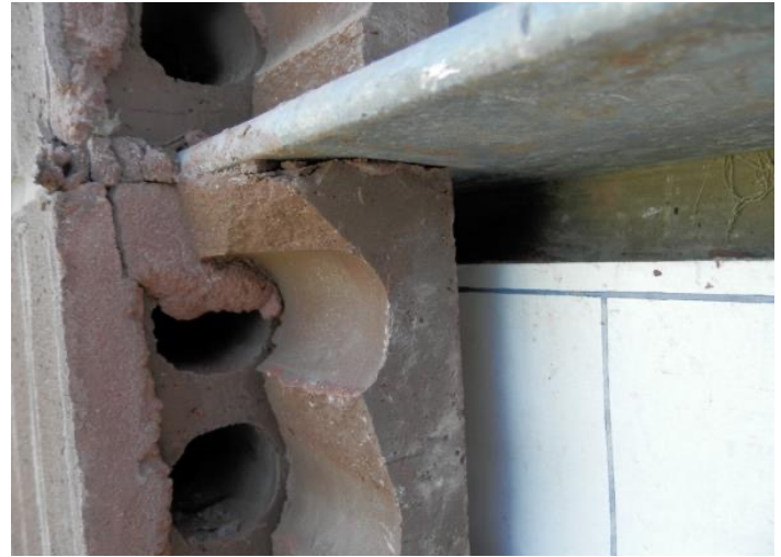
PHOTOGRAPH 10. A view of the steel shelf angle below a horizontal crack. Photo from Rimkus Archives.
