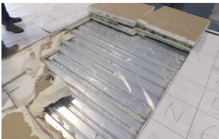
FIGURE 7. Destructive testing upon completion of a test to evaluate the mode of failure.
