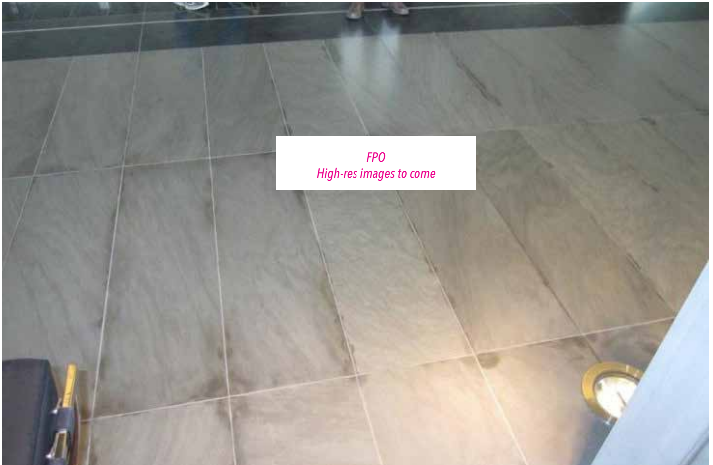
FIGURE 1. Permanently stained interior flooring from moisture exposure.
