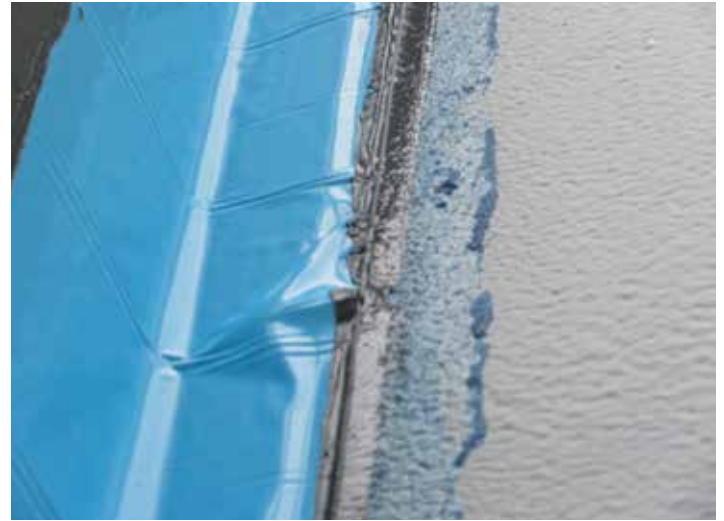
Figure 16. Photo of fishmouth and loose area of self-adhering flashing applied over fastener head.
