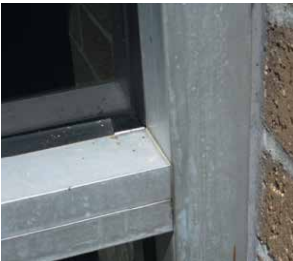
Figure 13. Photo of gap between ends of abutting gaskets at interface of vertical and horizontal mullions.
