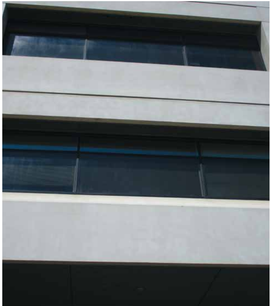
Figure 19. Photo of sealant joints in wall panels intersecting joint around window frame.
