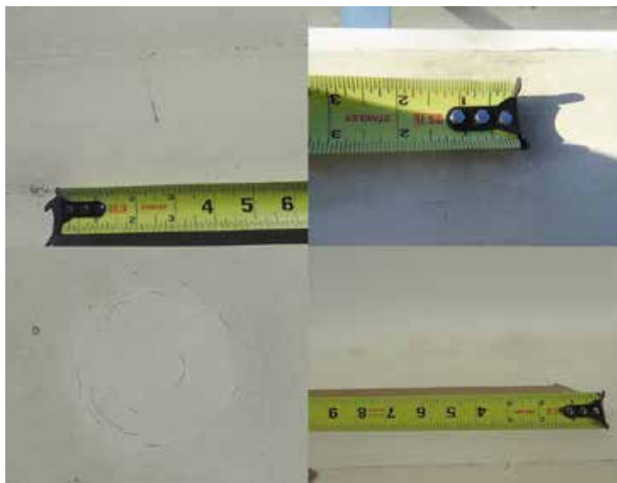
Figure 5. Typical arc-shaped fractures at back of a seam (upper left), back of an edge metal flashing (upper right), a cover board fastener plate (lower left), and roof-to-wall corner bend (lower right).
