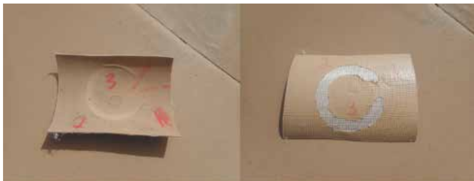
Figure 4. Pinch-type/"anvil strike" hail fracture on a membrane test cut, marked "3," visible on both top and bottom surfaces of membrane. Note that while the surface fracture marked "1" on the membrane is visible as an indentation on the bottom of the membrane, no actual separation of the membrane's underside was present at this location.
