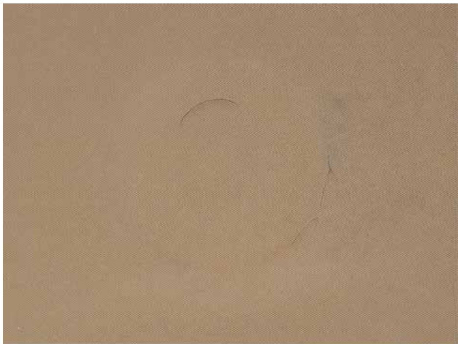
Figure 2. Arc-shaped fractures that interrupt each other at a fastener plate.
