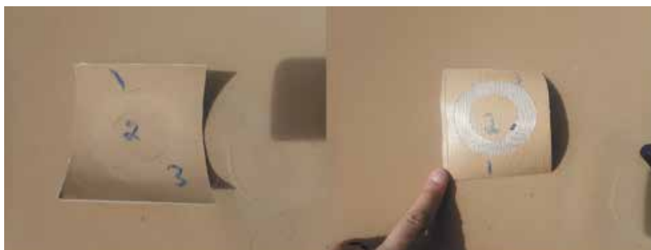
Figure 3. Test cut at fastener plate; note fractures not present on membrane underside.
