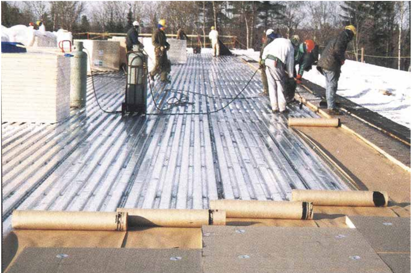
Figure 4. Forty years ago, kraft paper may have been applied directly to a steel deck in bituminous adhesive as the vapor control layer. The vulnerability to puncture is clearly evident. Accordingly, a hardboard layer should first be installed over fiber-reinforced polymer prior to vapor retarder application.
