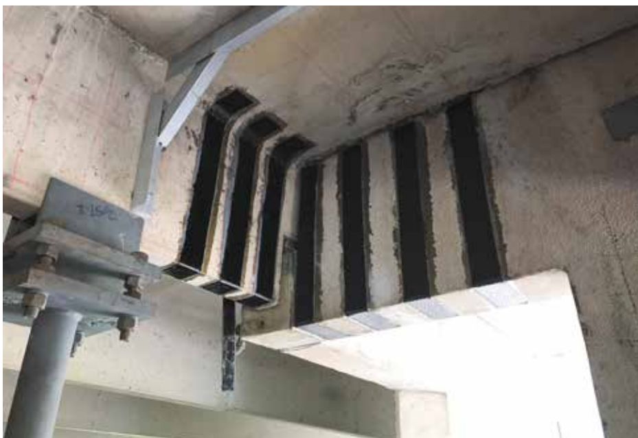
Figure 1. The strength and versatility of fiber-reinforced polymer have long been recognized. Here, carbon-fiber wrap is being deployed during extensive repairs to a parking deck.
