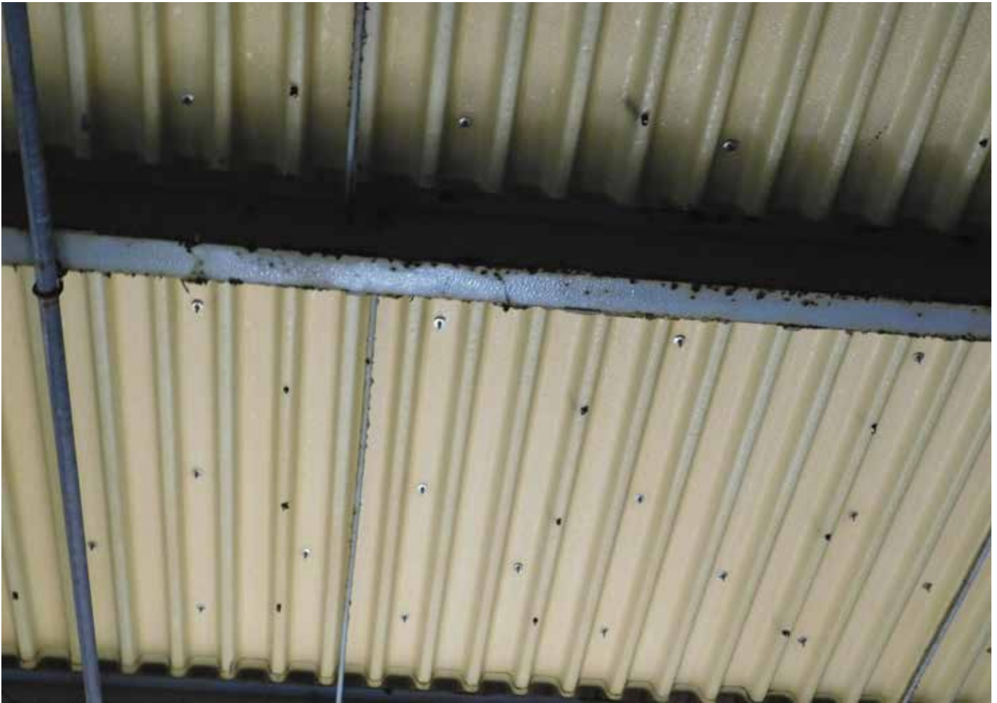
Figure 5. This old fiber-reinforced polymer deck had electrical conduits improperly situated over the supports. Notice the line of sidelap stitching screws and the specialty fasteners used to secure roof insulation (Image courtesy of Teamcraft Roofing, Salisbury, NC).
