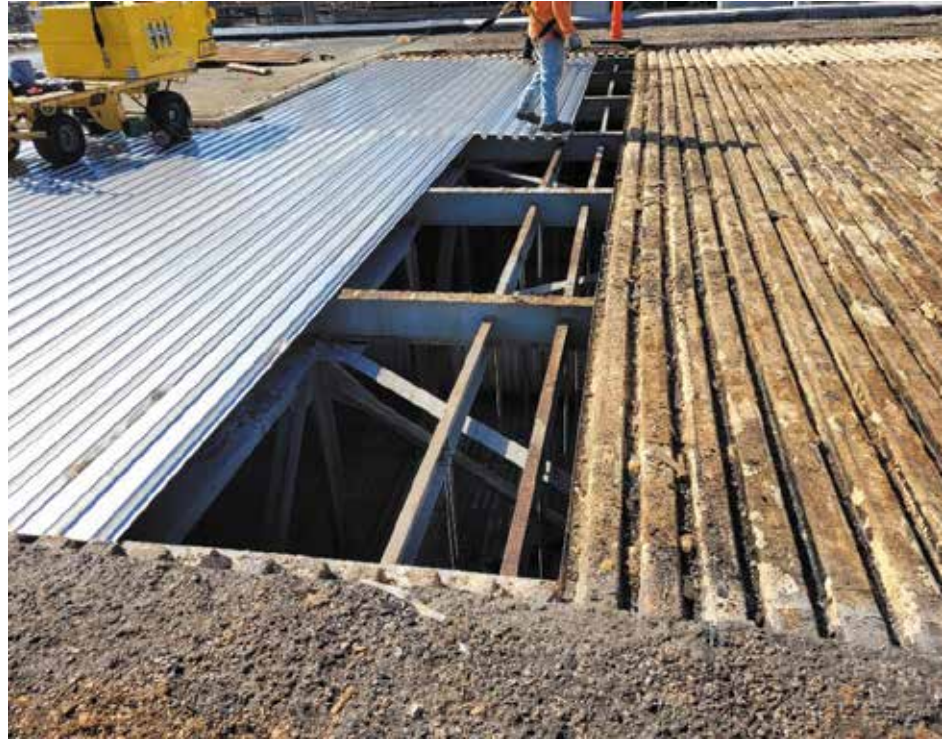
Figure 2. Old built-up roofing and decades-old fiber-reinforced polymer deck in a corrosive environment being replaced here with new stainless steel decking (Image courtesy of Teamcraft Roofing, Salisbury, NC).
