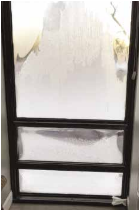
Figure 5. Condensation at a concrete-frame building in a cold climate.
