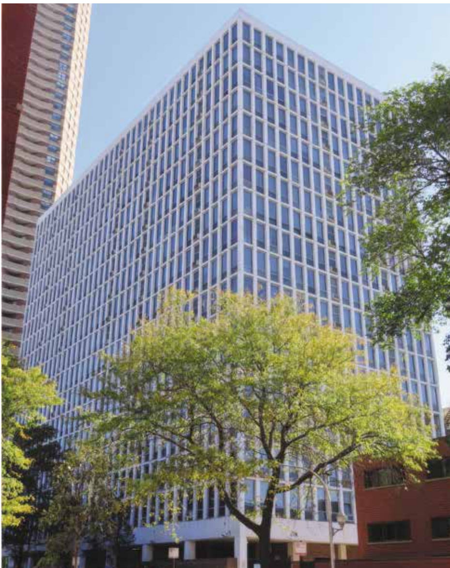
Figure 1. Building exterior walls consisting of concrete columns, concrete slab edges, windows, and sealant joints.
