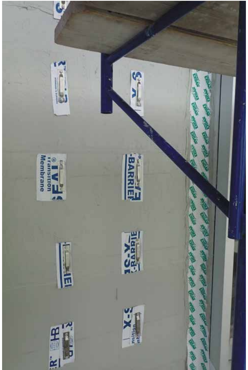
Figure 7. Installation of new sheathing, air barrier, and brick ties during masonry reclad.
