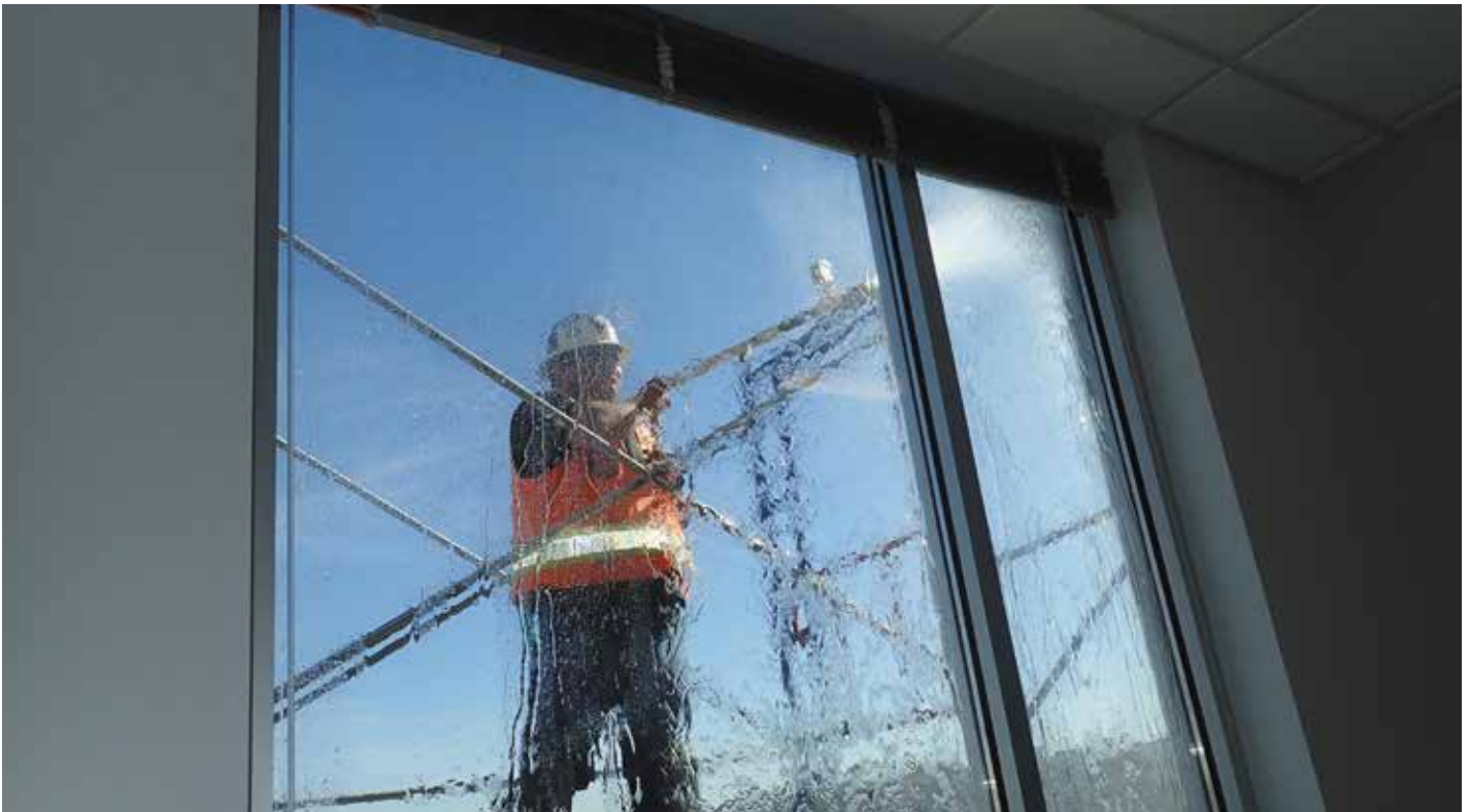
Figure 9. AAMA 501.2 nozzle water testing was performed at a punch window in order to evaluate potential water leakage.
