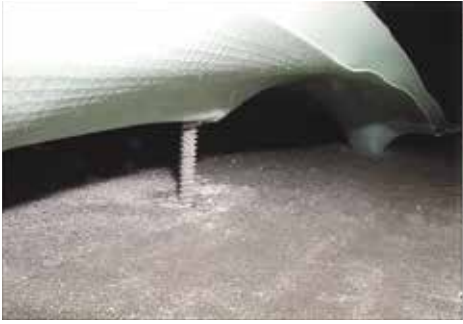
Figure 10. Fastener pullout from the steel deck.
