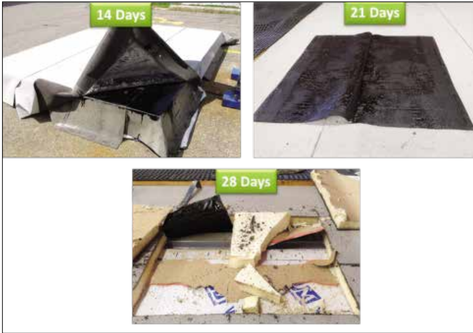
Figure 22. Failure modes varied with curing time for an adhesive applied membrane roofing system.
