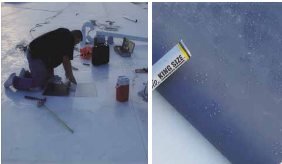
Figure 23. Condensation below the roof membrane.
