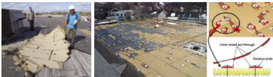
Figure 15. Substrate pullout from the fastener and plate for a partially attached (hybrid) membrane roofing system.
