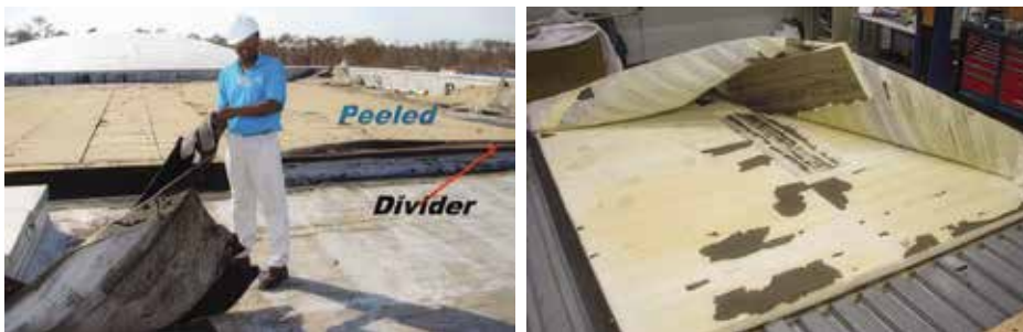
Figure 16. Facer delamination failures for an adhesive applied membrane roofing system.
