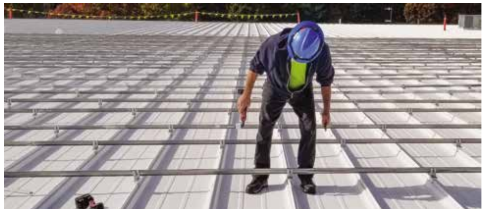
Figure 1. Flush Rail Mounting; Use of rails on the metal roof is redundant and adds unnecessary collateral load.
