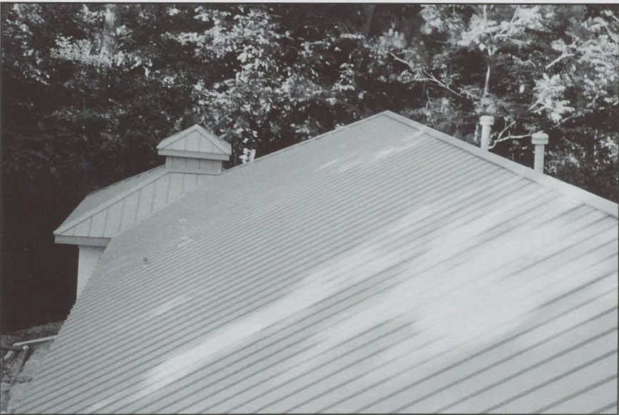
Standing seam roof on architect's home in Houston, Texas, was completed in May of 1995.
