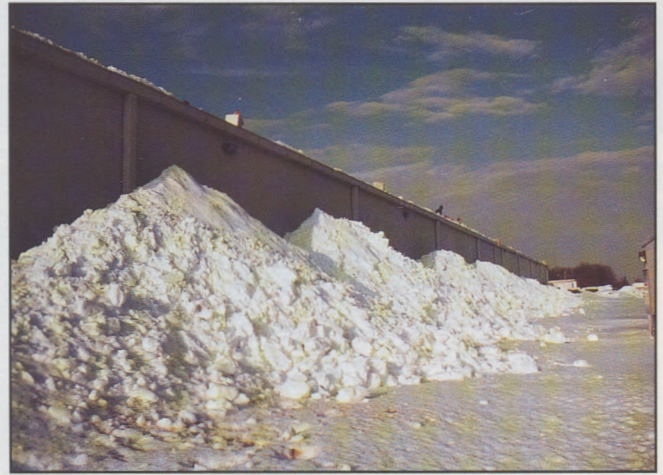
Piling snow alongside a building can cause wall damage.
