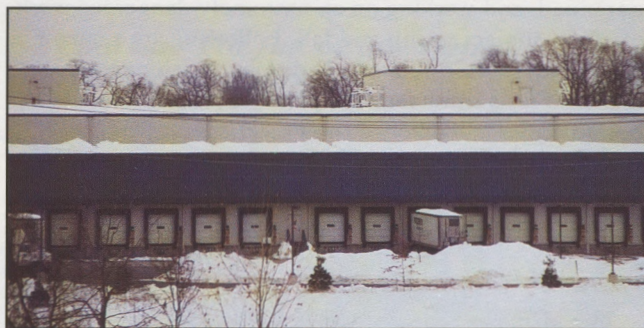
Note drainage channeling from the high to the low roof to allow water melt to roll into gutter edge along front.
