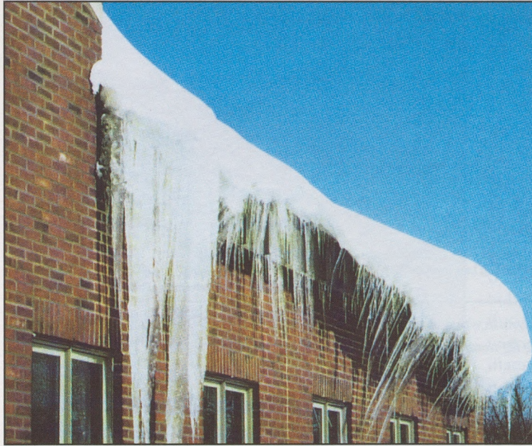
Figure 7: Icicles will form on an overhanging, creeping mass of ice and snow.
