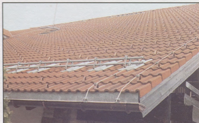
Metal snow brackets on a tile roof in the German Alps.
