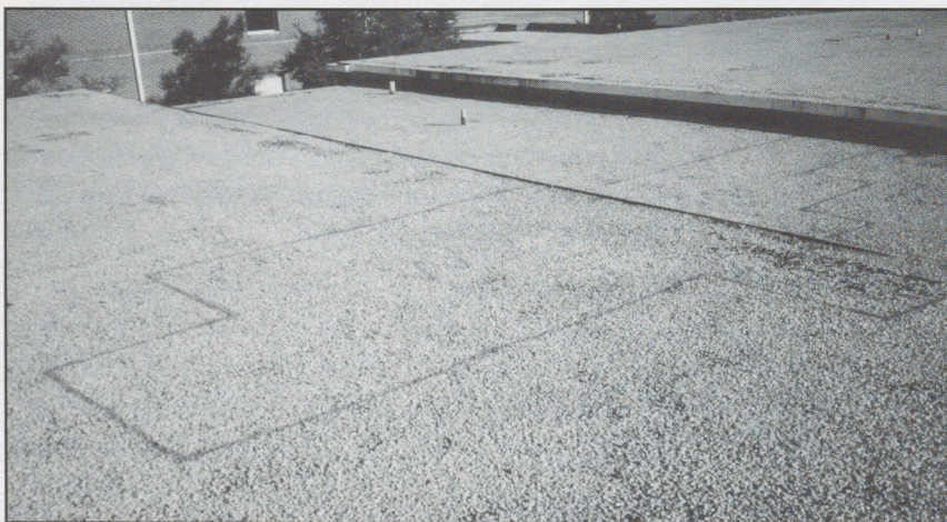
Suspected "wet" area delineated on the roof surface.
