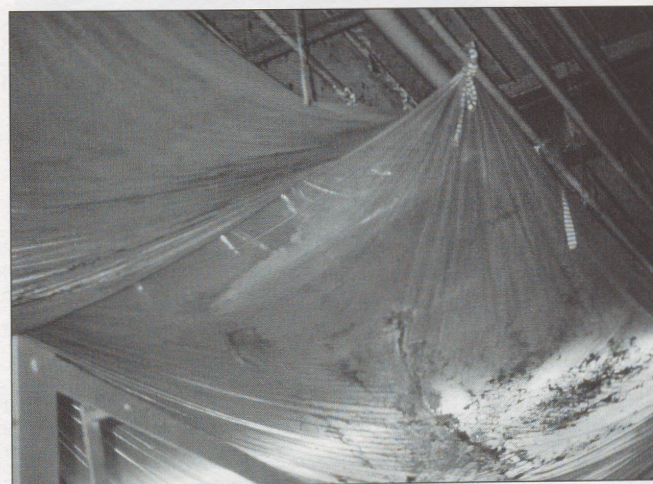
These photos show a few examples of what can fall as a result of vibration caused by work being conducted on the roof or just from leaks. Ceiling tile and pipe wrap often contain asbestos.
