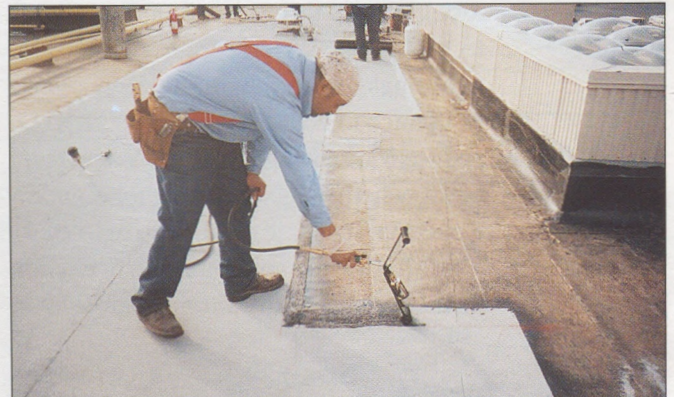
Installer heating granule surfacing at end lap of bottom sheet prior to applying overlying sheet.
