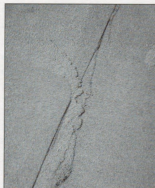
Granules embedded in asphalt bleed-out and rounded corner of end lap.
