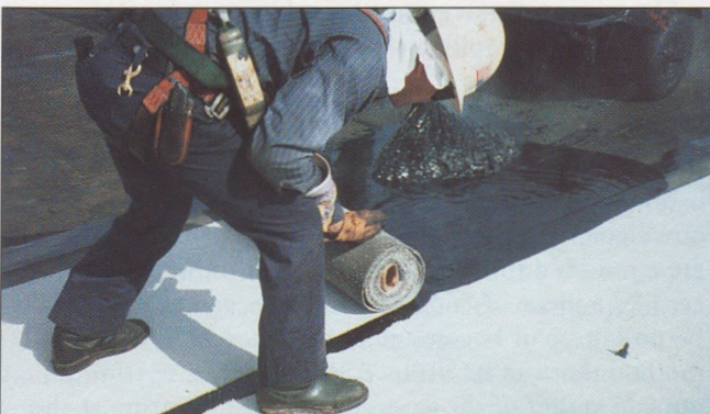
Installer applying downward pressure on cap sheet roll while maintaining roll in close proximity to asphalt mopping source.
