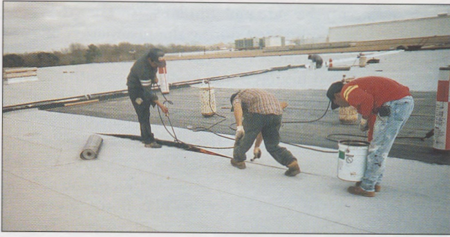
Fusing the side laps of a torch-applied modified bitumen cap sheet utilizing hand-held torching equipment, rolling the heated seam and embedding granules into the bleed-out.
