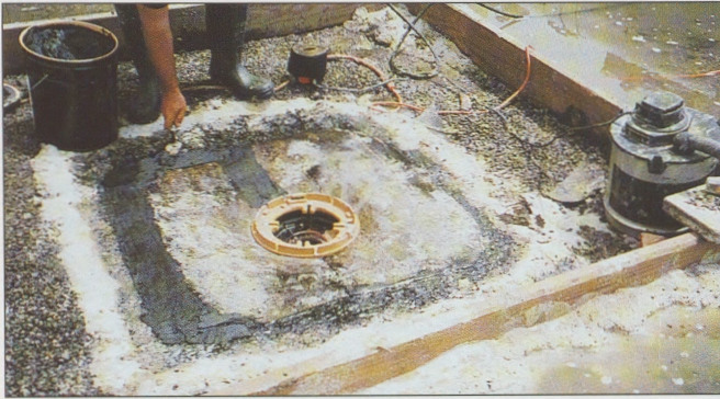
A coffer dam was built in 4"-deep water. A new relief drain was installed and flashed into the existing pitch roof membrane.
