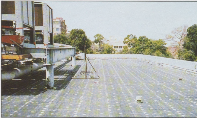
The venting base sheet has been fastened with base ply fasteners with 1-90 plates.
