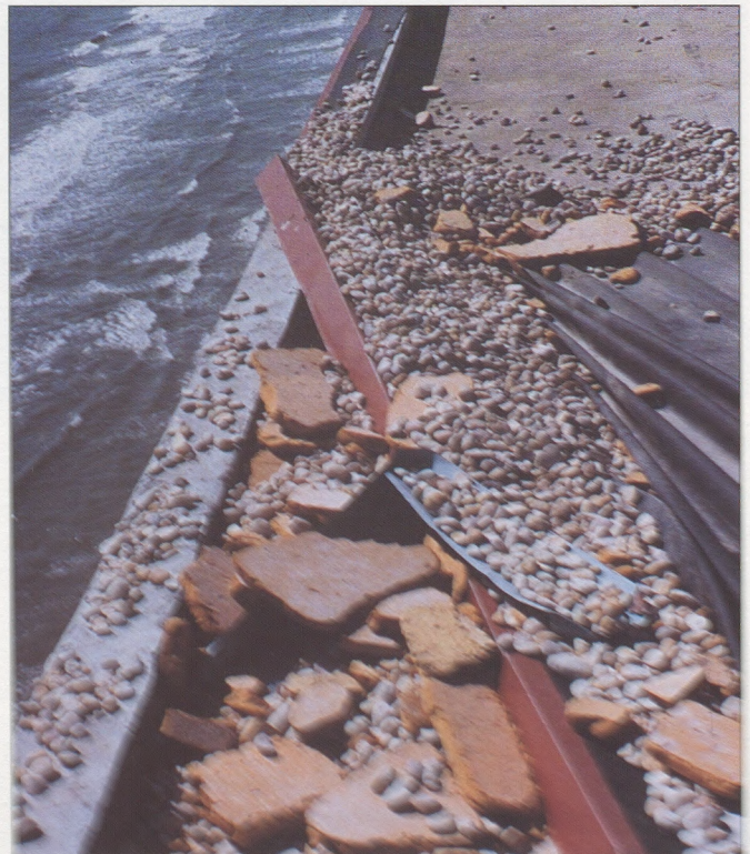
The edge detail on this roof failed, resulting in membrane failure at the perimeter during Hurricane Hugo.
