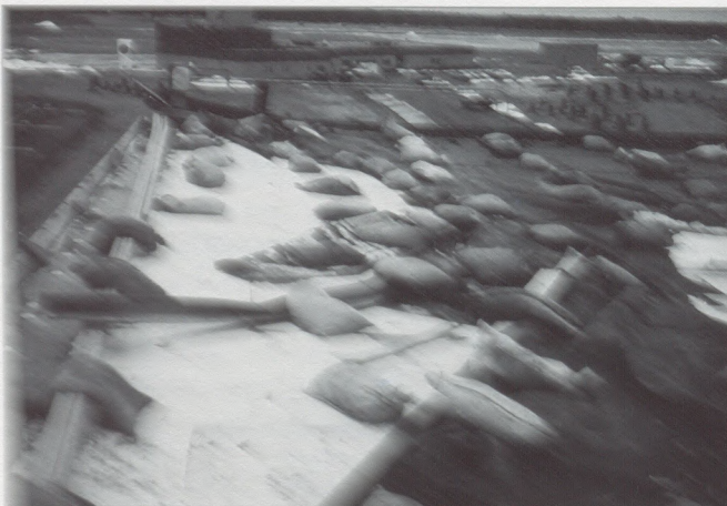
Photo 1: Wind damage to a fully-adhered single-ply membrane.
