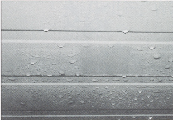
Photo 3: Condensation on the underside of standing seam metal roofing.
