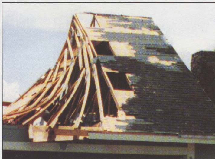
Figure 9: Progressive failure of truss system from inadequate lateral bracing. Photo courtesy of RCI.
