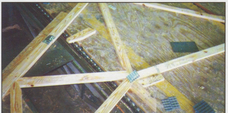
Figure 6: Metal plate-connected wood truss being assembled on the truss manufacturing table (jig). Photo courtesy of Blue Ox Industries, Inc., Kernersville, NC, (800)-672-2145.
