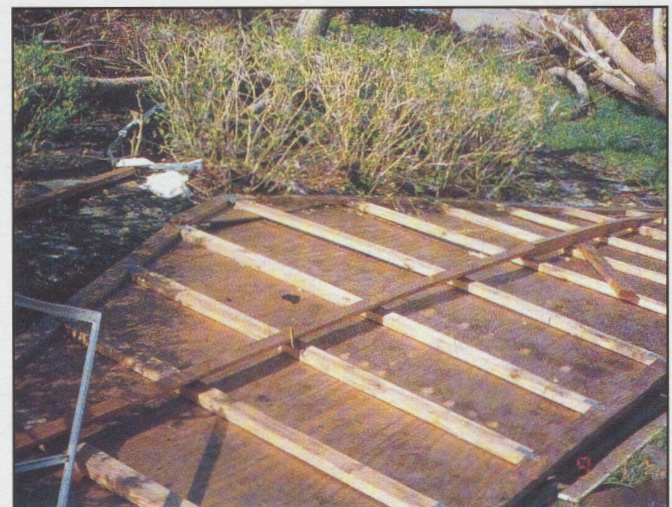
Figure 13: Loss of entire endwall during windstorm. Photo reprinted courtesy of FEMA, Washington, DC.
