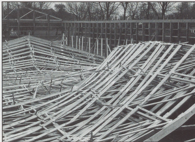
Figure 8: Use of "killer cleats" as installation bracing can lead to truss collapse such as this. Photo courtesy of Wood Truss Council of America.
